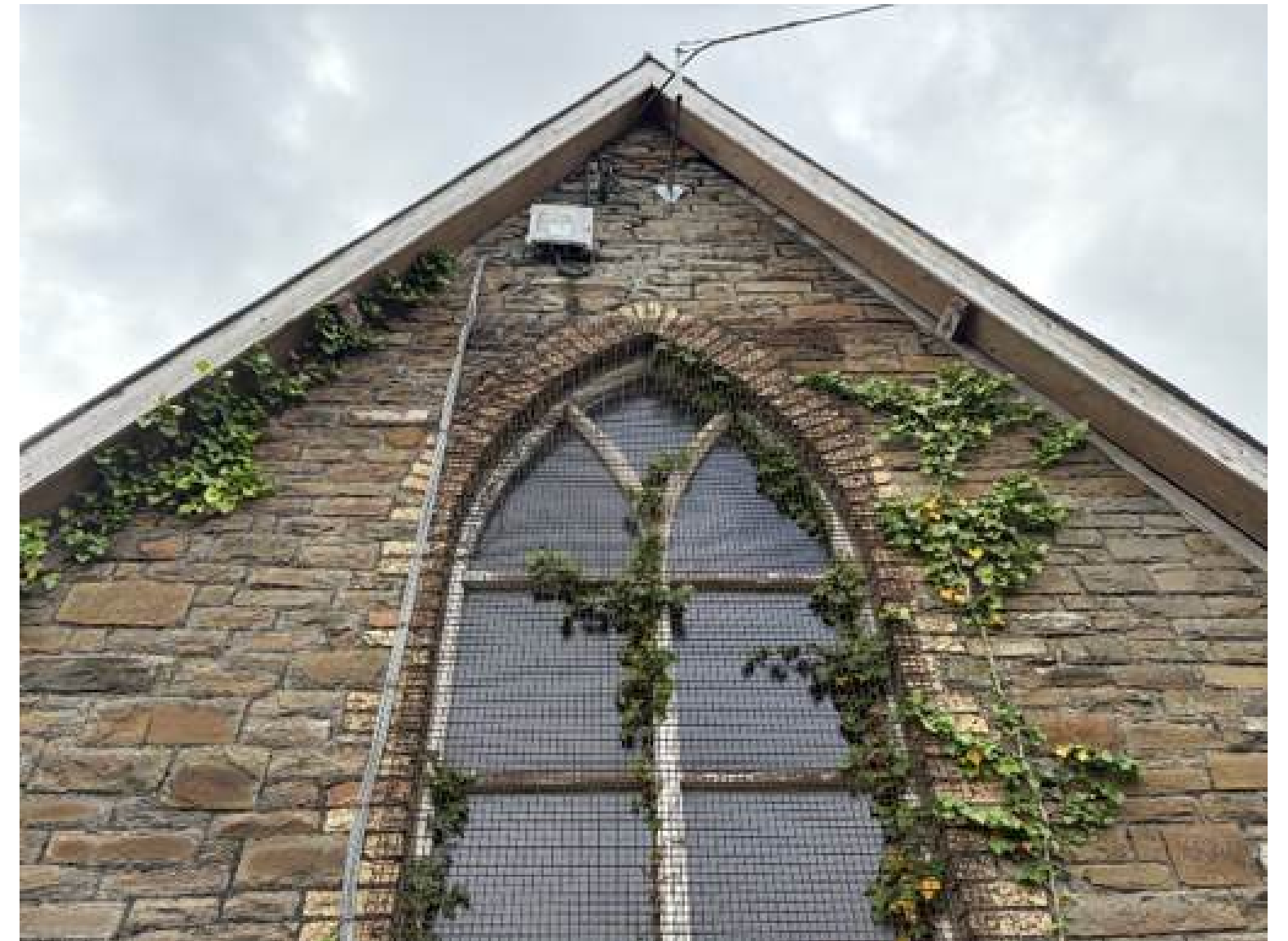
Figure 20 - Foliage growth, missing pointing
