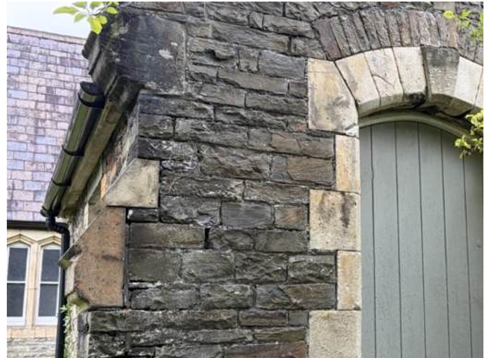
Figure 18 - Missing lime pointing
