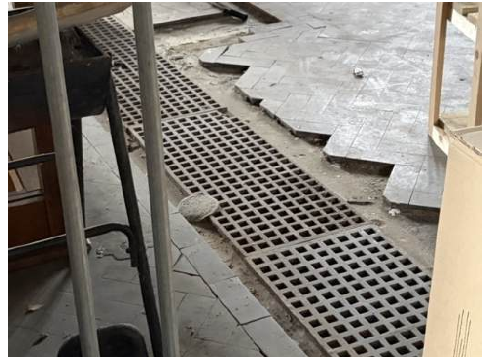
Figure 26 - Missing parquet floor
