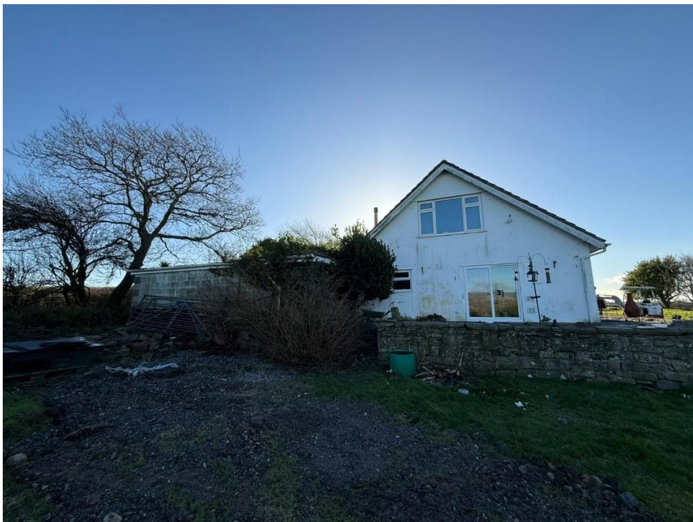
Figure 4: Side elevation and view of garage (Flat roof has been replaced due to storm damage)
