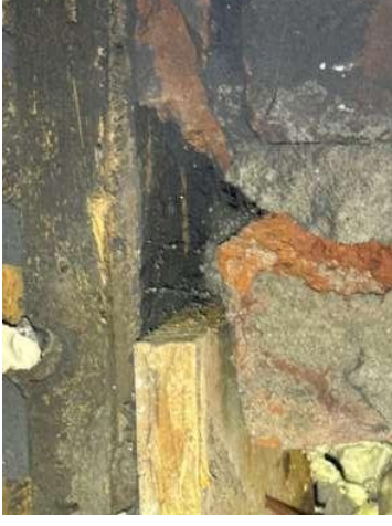
Mortar gap in the newly exposed brick walls.
