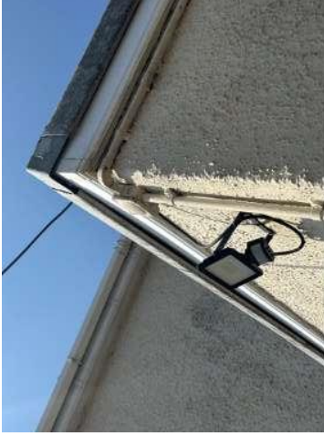
Slight gap under flat roof felt and barge board.
