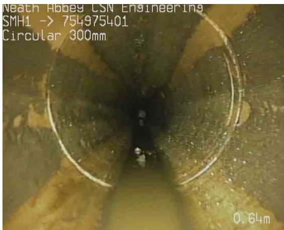
1, 00:00:19, 0.81 m Crack, circumferential from 1 o'clock to 5 o'clock
