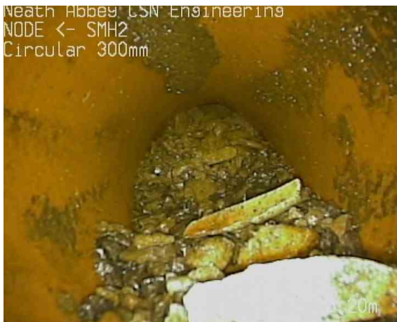
1, 00:00:13, 0.20 m Settled deposits, fine, 30% cross-sectional area loss
