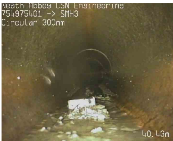
3, 00:03:33, 40.43 m Settled deposits, fine, 5% cross-sectional area loss
