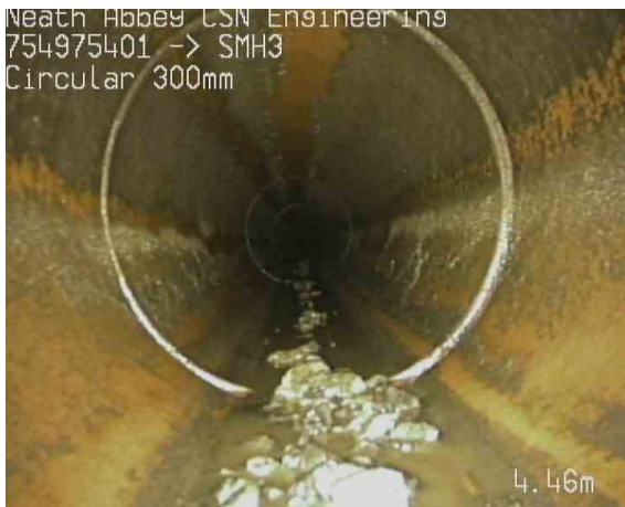
1, 00:00:41, 4.46 m Settled deposits, fine, 5% cross-sectional area loss
