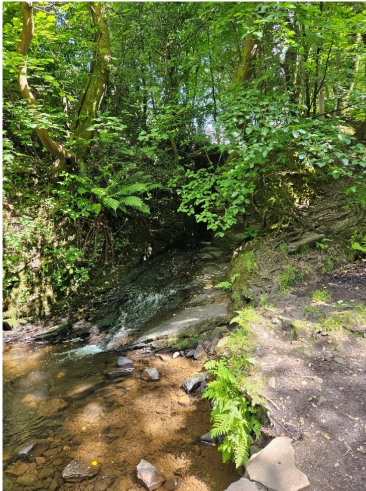
Figure 5-7 – Erosion damage to the Railway Incline resulting from the Grandison Brook, to the south of the playpark in Jersey Park.
