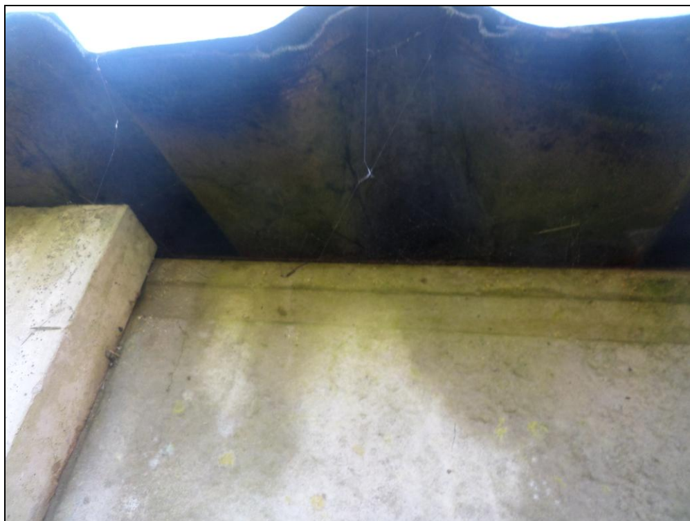
Photo 8: Gaps beneath corrugated roof providing access to interior.
