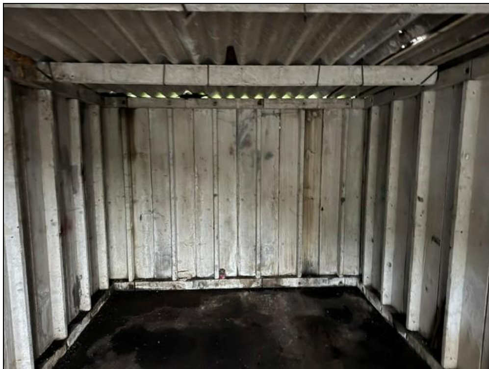
Photo 11: Interior of garage with exposed asbestos roof.
