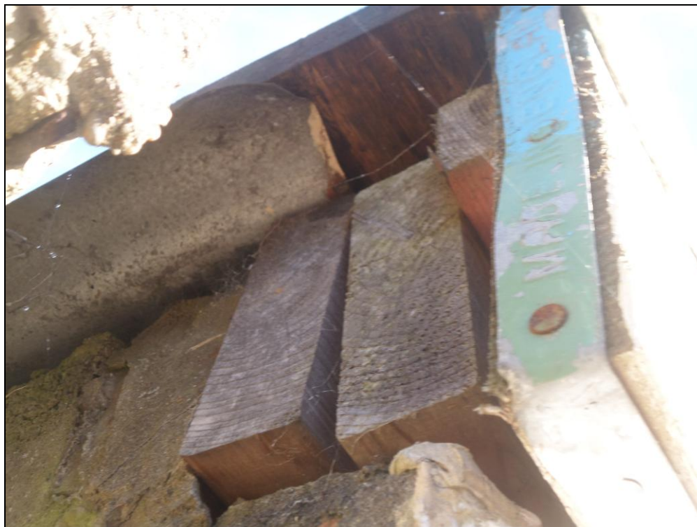
Photo 9: Gaps beneath fascia on detached easternmost garage.
