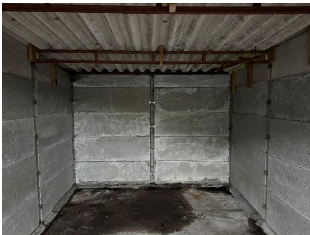
Photos 10: Interior of garage with exposed asbestos roof.
