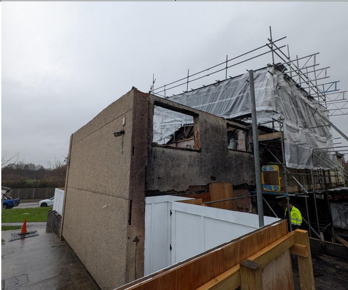
Photograph 1: Existing fire-damaged dwelling on site.
