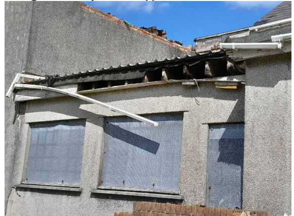
Image 5: Gaps in soffit - side extension
