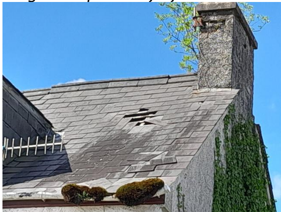
Image 3: Gaps in roof - front elevation
