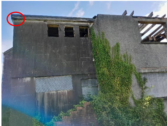
Image 7: Openings and soffit gaps on rear elevations. House sparrow nesting site indicated
