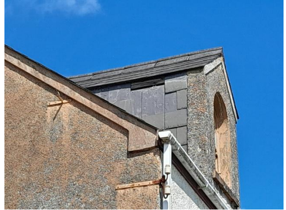
Image 4: Gaps in side of dormer
