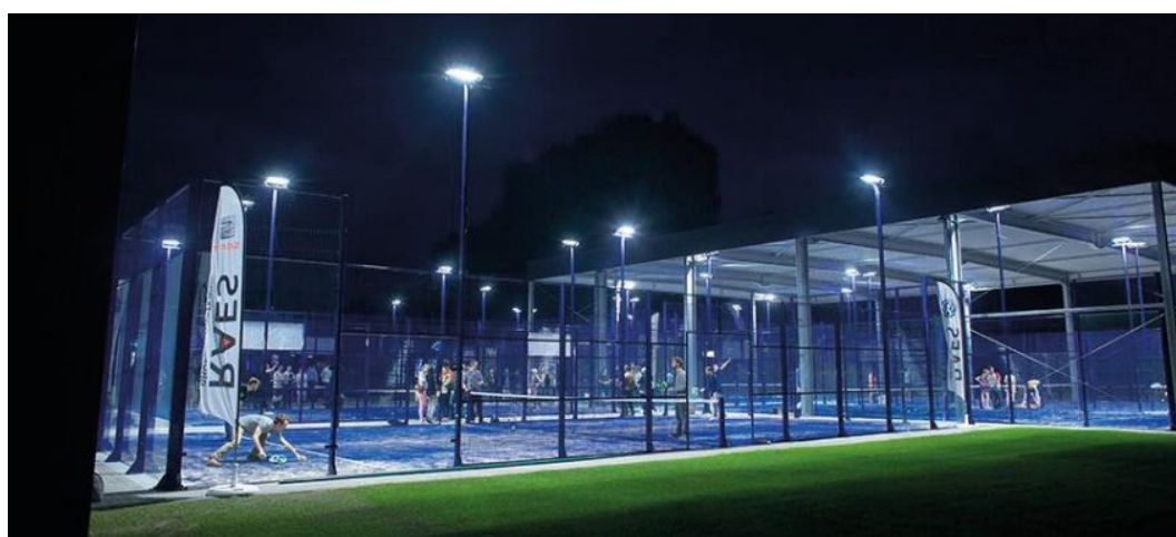
Figure 2 - Example of Fence Mounted Luminaires
