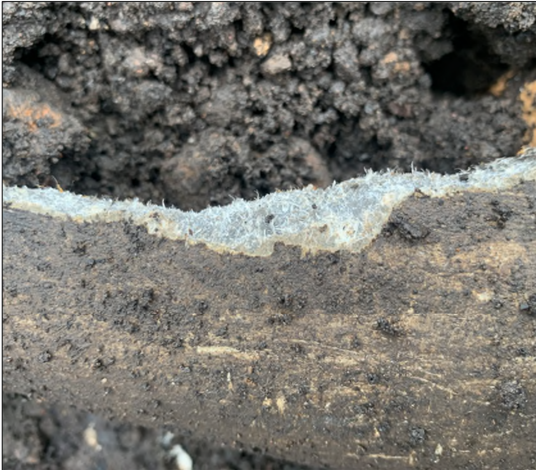
Figure 4.1 Segment of asbestos pipe located at a depth of 0.4m in TP03.
