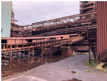
No5 Charging Conveyors
