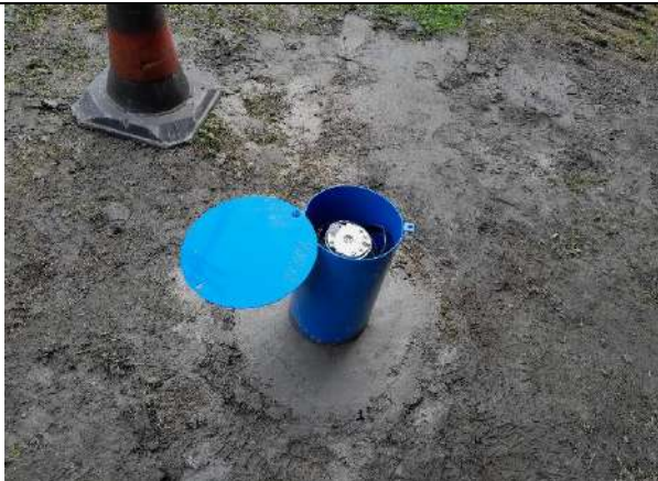
4. Instrument deployed in raised headworks.
