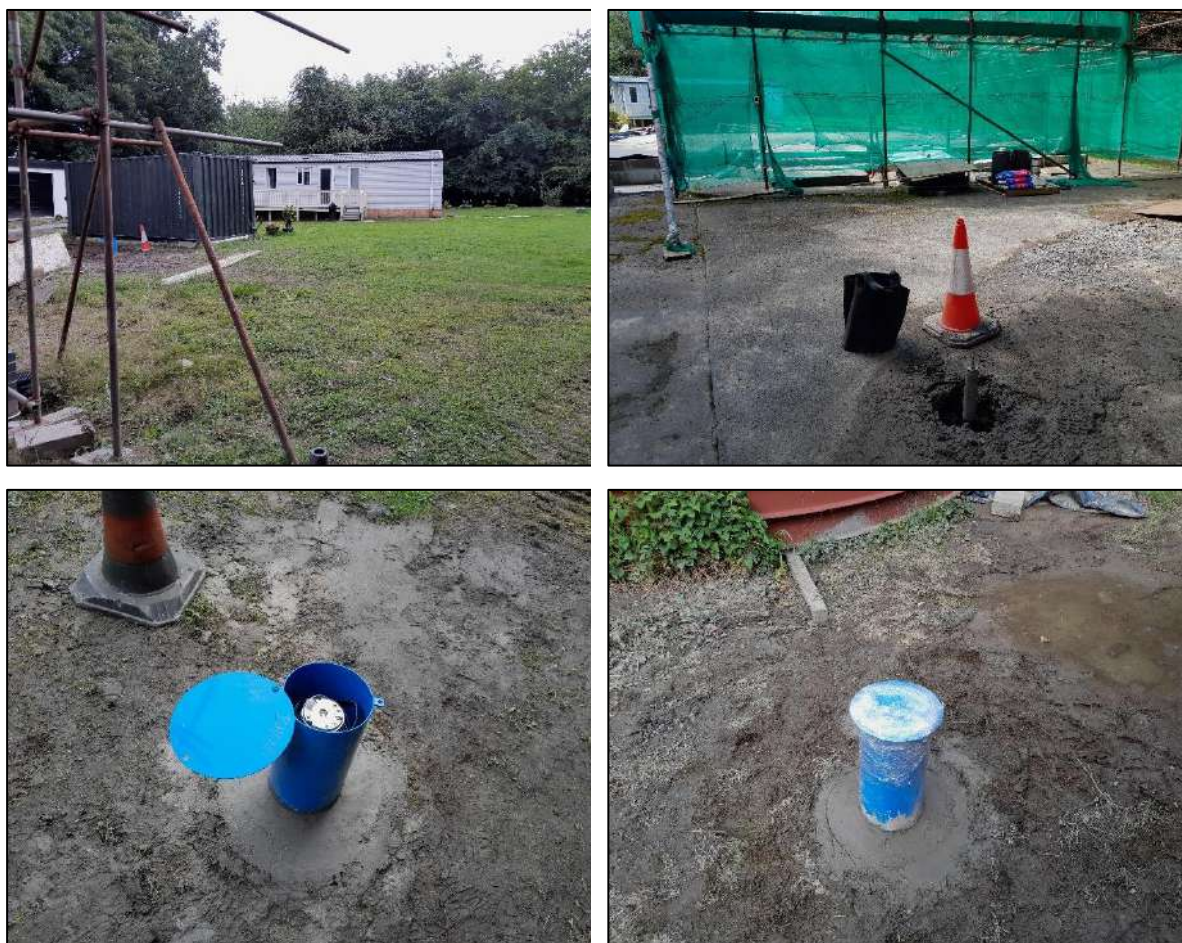
Figure 1 Selected GGS site photographs (July 2025). Image top left: general site photograph. Image top right: monitoring well before GGS headwork installation. Image bottom left: continuous monitoring instrument deployed. Image bottom right: headworks secured.
