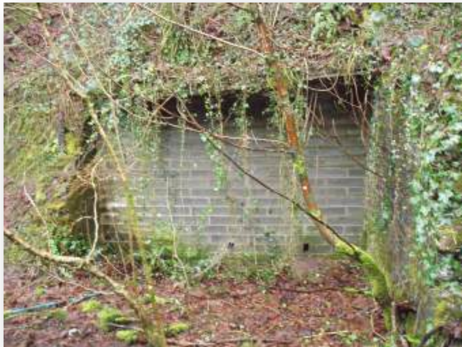
Figure 12 The Blocked Up Entrance of Adit 277209-058
