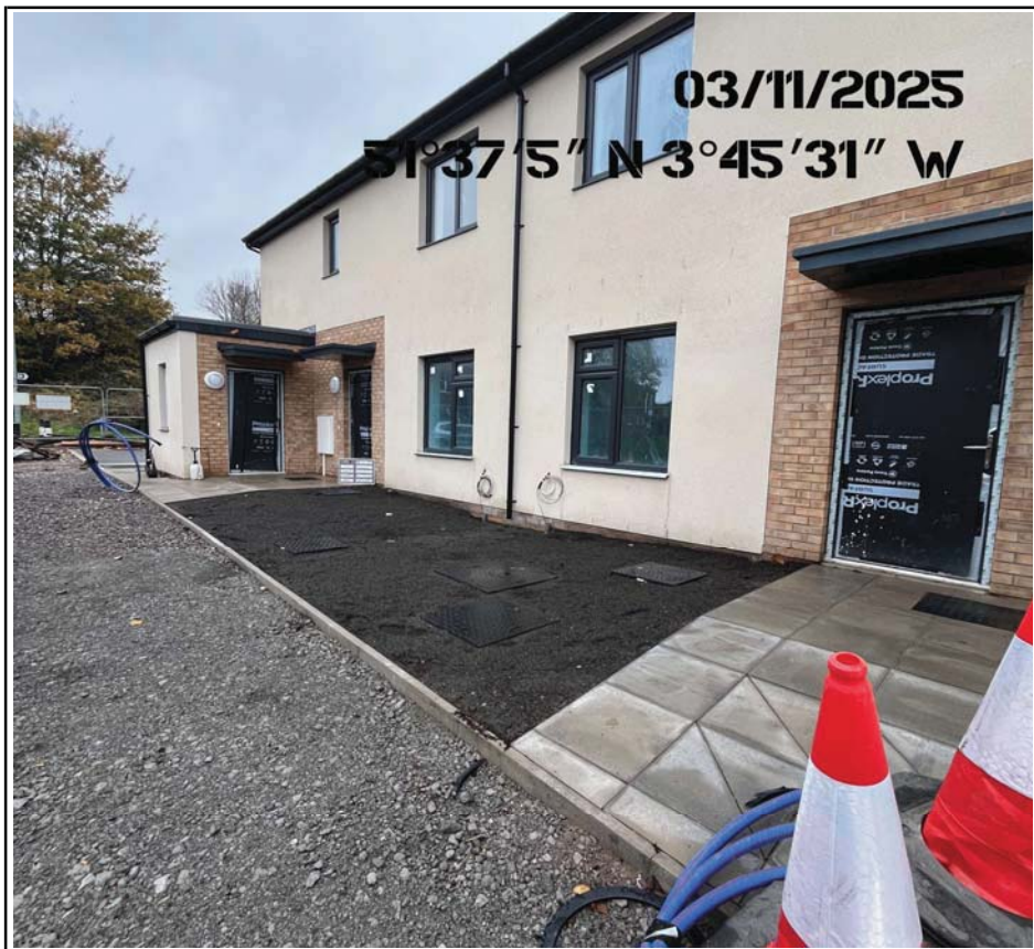
Plot 40 to 43 Rain Garden System Area
