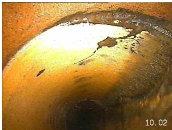
6, 00:03:50, 10.02 m Fracture, spiral at joint from 1 o'clock to 3 o'clock
