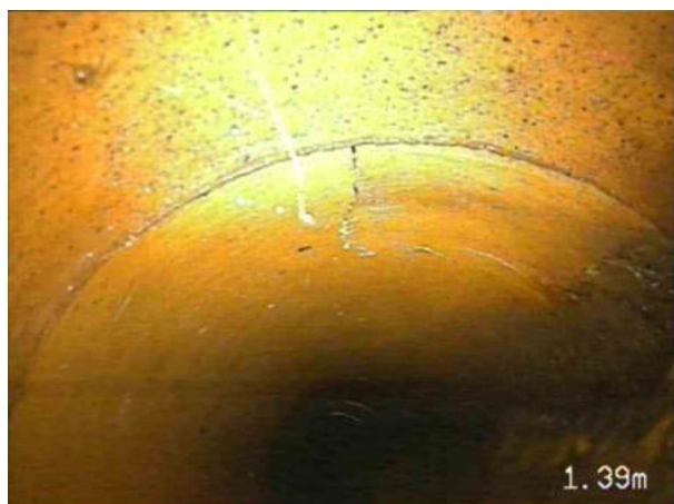
1, 00:00:46, 1.39 m Fracture, longitudinal at joint at 4 o'clock
