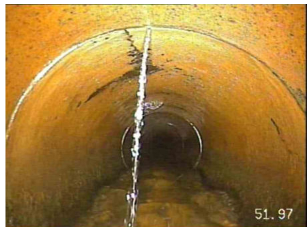
12, 00:13:56, 51.97 m Infiltration, running at 12 o'clock
