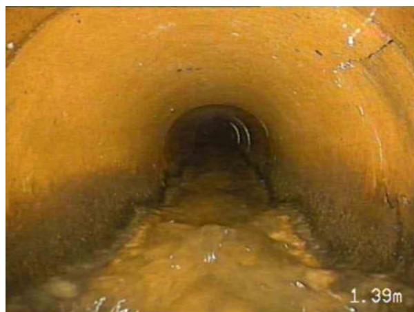
2, 00:00:52, 1.39 m Fracture, longitudinal at joint at 2 o'clock
