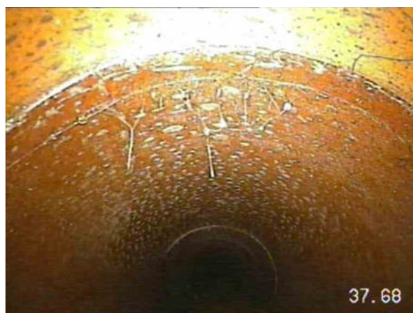
4, 00:06:18, 37.68 m Fracture, spiral at joint from 10 o'clock to 2 o'clock
