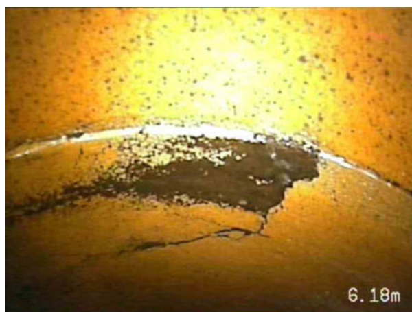
4, 00:02:32, 6.18 m Fracture, spiral at joint from 8 o'clock to 10 o'clock
