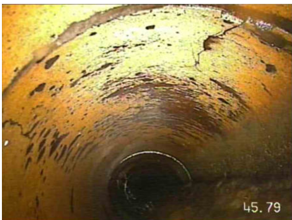
11, 00:12:27, 45.79 m Fracture, longitudinal at joint at 3 o'clock
