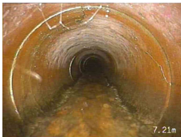
2, 00:01:25, 7.21 m Fracture, longitudinal at joint at 12 o'clock
