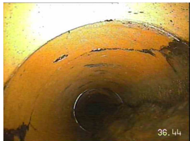
10, 00:10:36, 36.44 m Fracture, longitudinal at joint at 3 o'clock
