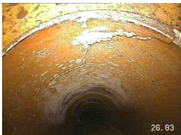
3, 00:04:00, 26.83 m Broken pipe at joint from 1 o'clock to 2 o'clock
