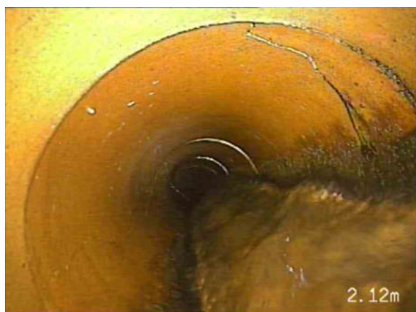
3, 00:01:10, 2.12 m Fracture, circumferential at joint from 2 o'clock to 4 o'clock
