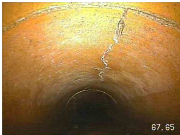
14, 00:16:59, 67.65 m Fracture, longitudinal at joint at 12 o'clock
