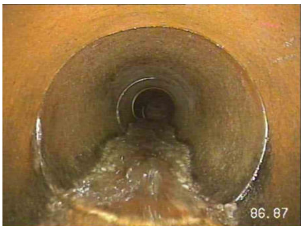
11, 00:14:29, 86.87 m Infiltration, running at joint at 9 o'clock
