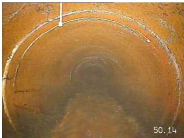
5, 00:08:21, 50.14 m Fracture, circumferential at joint from 7 o'clock to 2 o'clock
