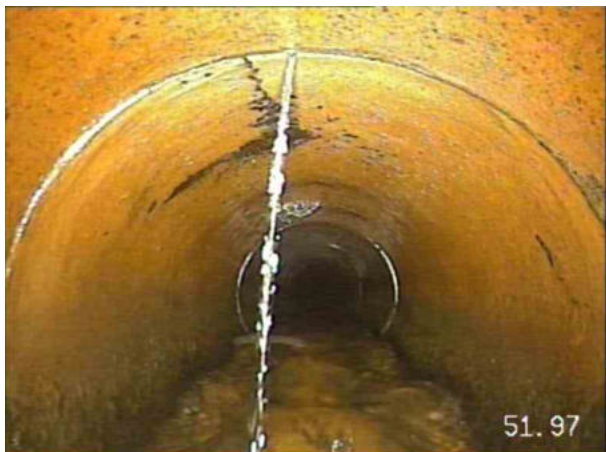
13, 00:13:59, 51.97 m Fracture, longitudinal at joint at 11 o'clock
