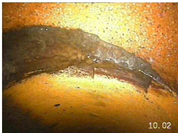
5, 00:03:33, 10.02 m Fracture, longitudinal at joint at 10 o'clock
