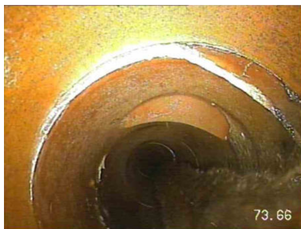
10, 00:12:56, 73.66 m Broken pipe at joint from 2 o'clock to 5 o'clock
