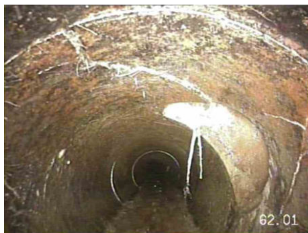
8, 00:10:50, 62.01 m Broken pipe at joint from 11 o'clock to 4 o'clock
