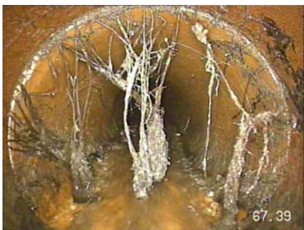
9, 00:11:58, 67.39 m Roots, mass, 10% cross-sectional area loss
