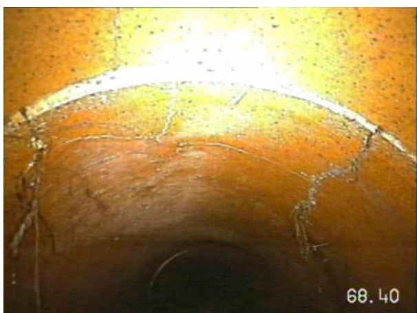
15, 00:17:40, 68.40 m Fracture, spiral at joint from 12 o'clock to 1 o'clock
