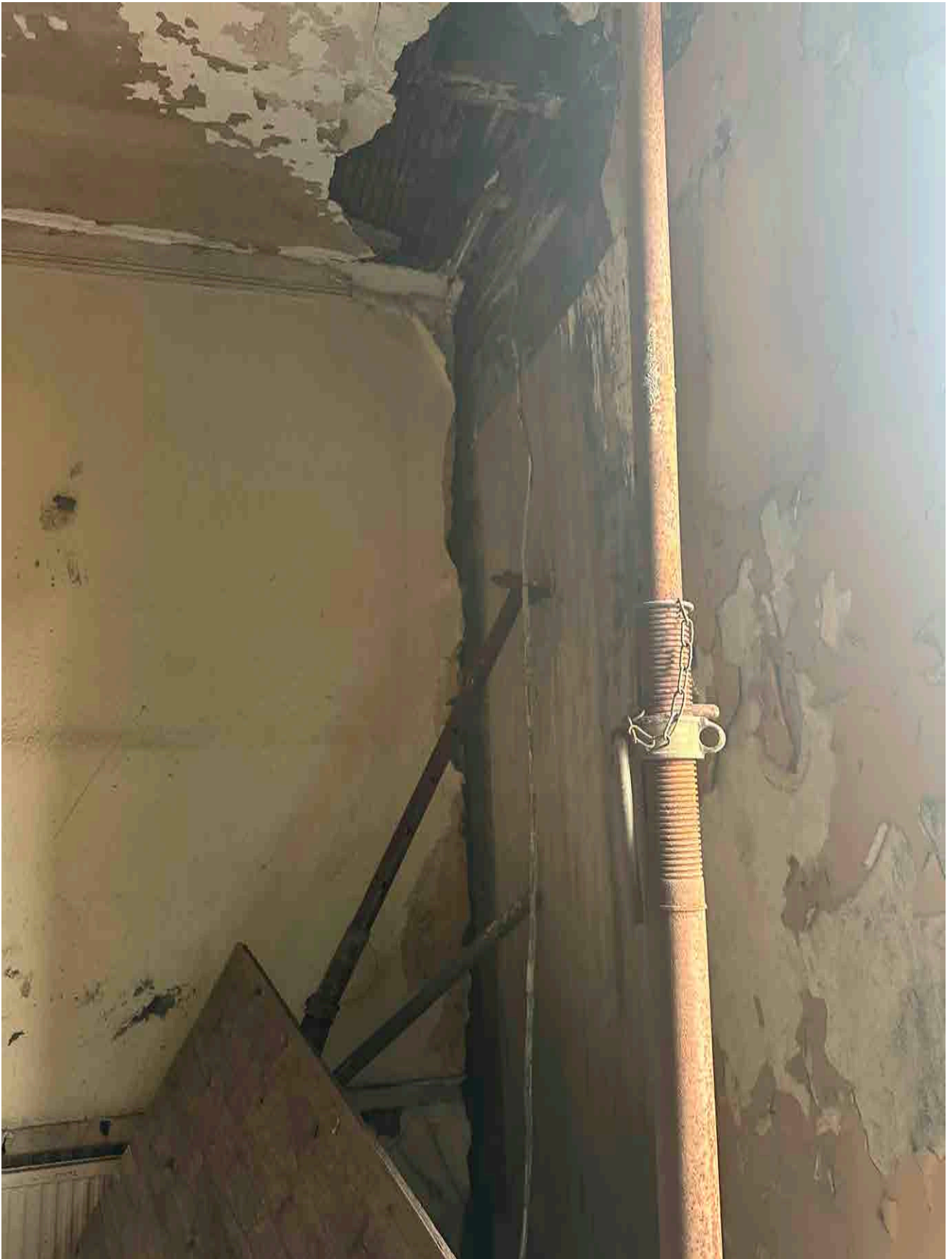
The front facade has become separated from a return wall inside the building
