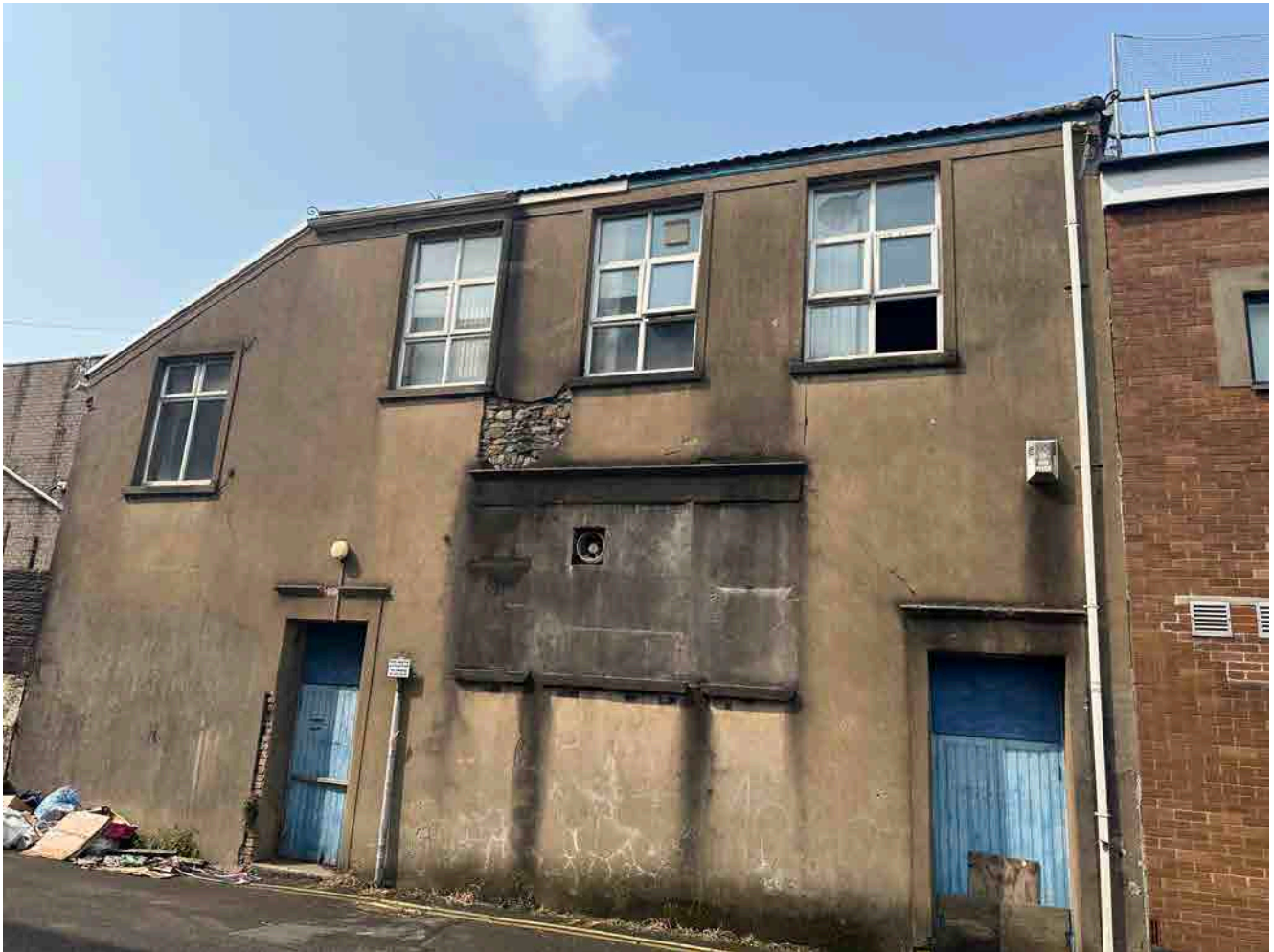
The rear of the building. Render has fallen off the wall in areas.
