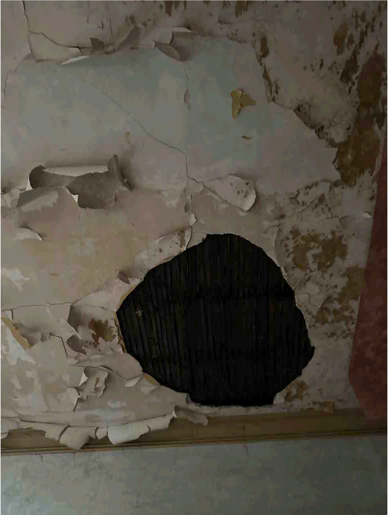
The first floor ceiling in the front section of the building is rotten and collapsed in some areas.
