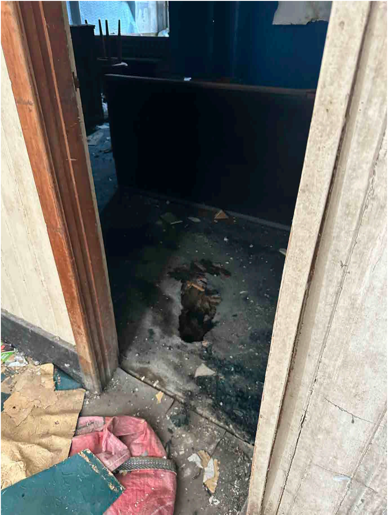
First floor in front section of the building. The timber is rotten and areas break underfoot
