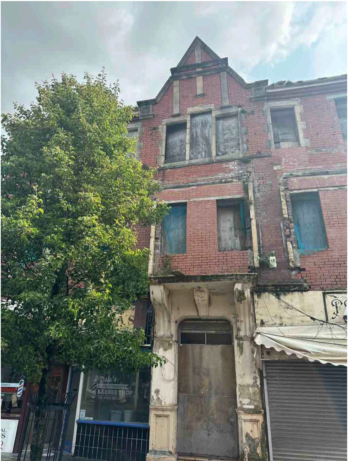
Front facade of the building. There are signs of bowing in the masonry panels.
