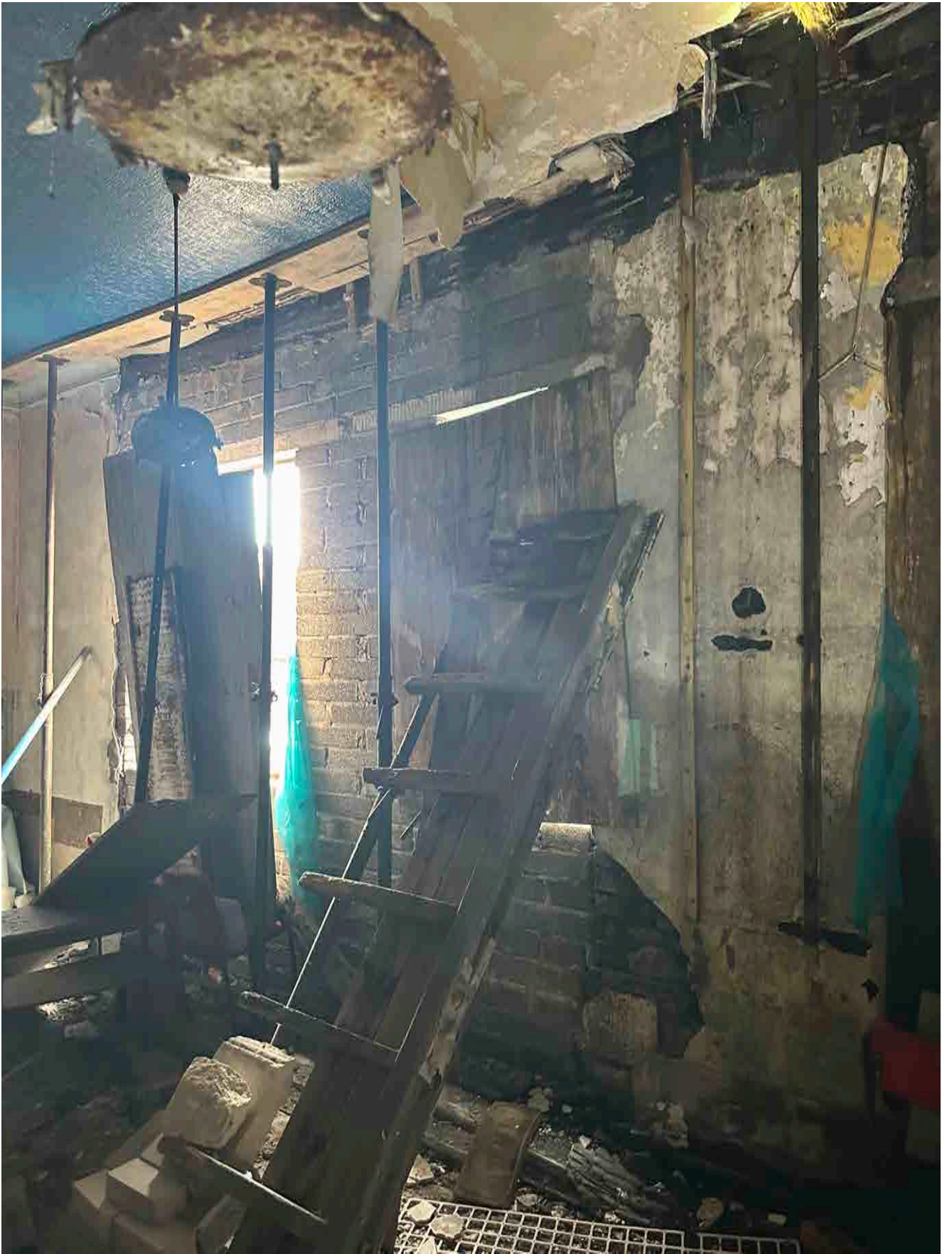
The interior face of the front facade. The floor above is propped as the timber sections have come a way from the facade in areas. The facade is leaning outwards.
