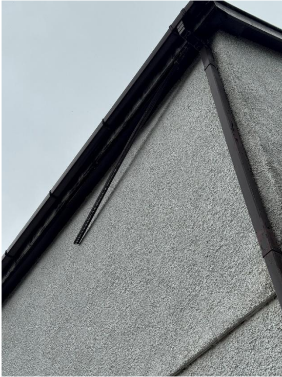
Plate 3 - Peeled back cladding on soffit board
