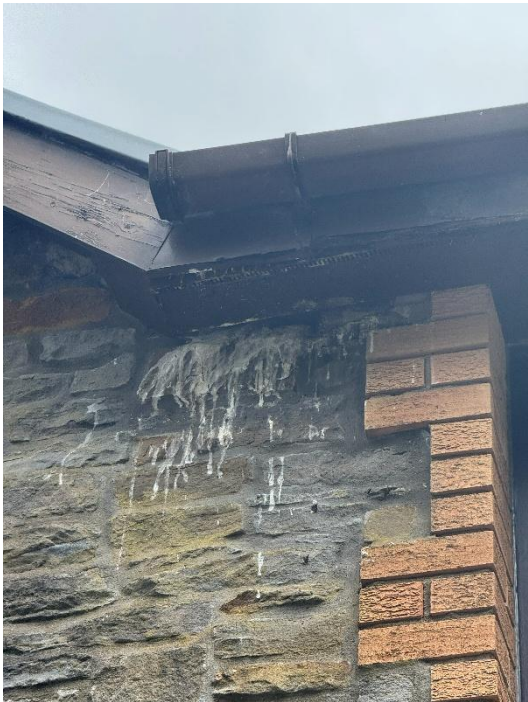
Plate 2 - Gaps under the soffit boards
