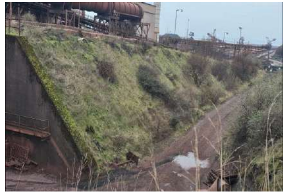
Fig.67 Ore Feeder ramp
