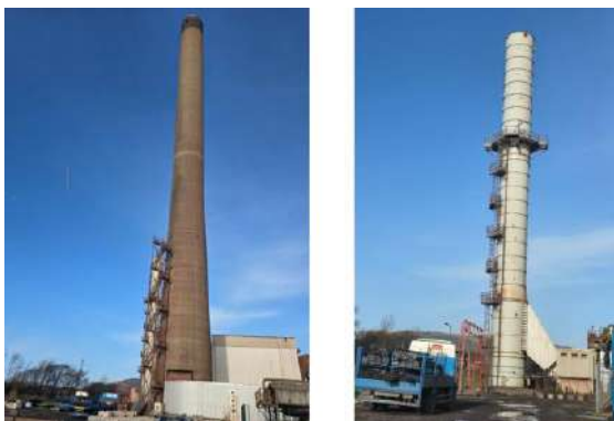
Fig. 18: Sinter Plant Concrete Stack (Chimney) & Secondary De-dusting Bag Filter Stack-Duct.
