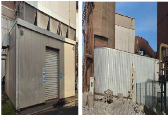
Fig. 17: De-Dust bag filter and Stack Ducting for Concrete Stack Tower room.
