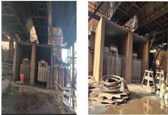
Fig. 16 : Transformer House Under Electrostatic Precipitators (DT 368, 367, & 366, 369).
