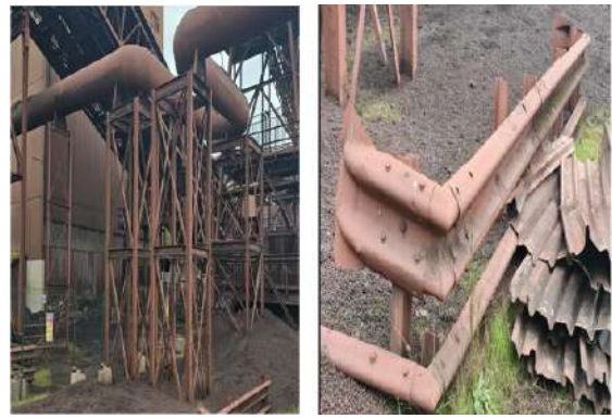
Fig.75: BOS pipeline support & Road barrier
