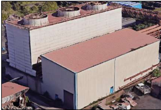
Fig.80: Cooling Tower & Pump
