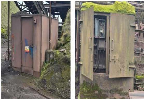
Fig.71 Electrical kiosk under Conv 731 and Electrical kiosk beside Conv 735
