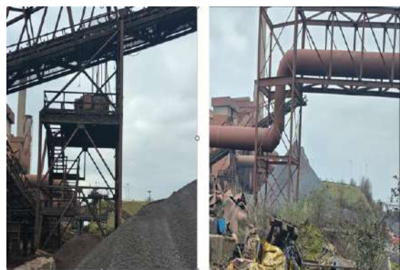
Fig.78: Conv 1028 support and Pipe bridge support LT156
