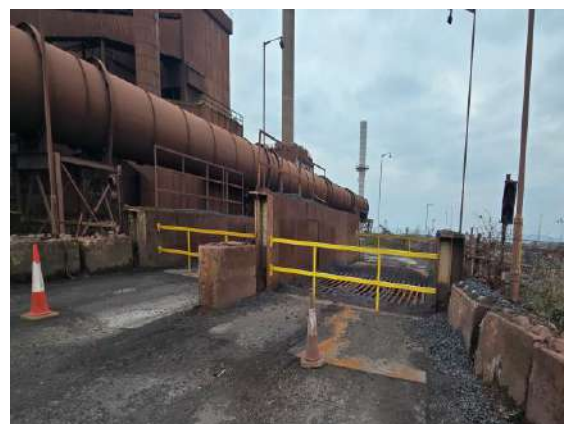
Fig.62: Ore feeder deck and screen
