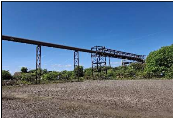
Fig.81: BOS Gas Pipe Line & Support
