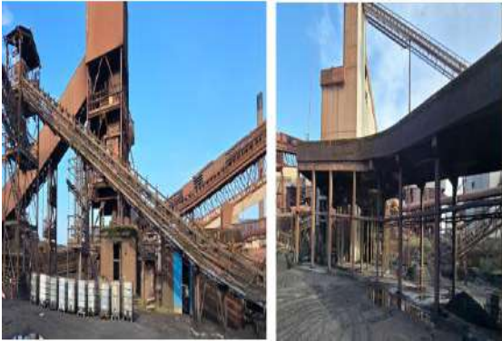
Fig.40 Conv 1089 and Concrete ramp.
