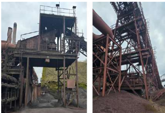
Fig.74: Junction house 731/735 & 727 & 735 GTU
