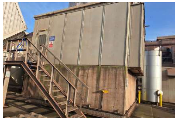
Fig. 22 : Centrifugal Fan-Soundproofing Cabin.
