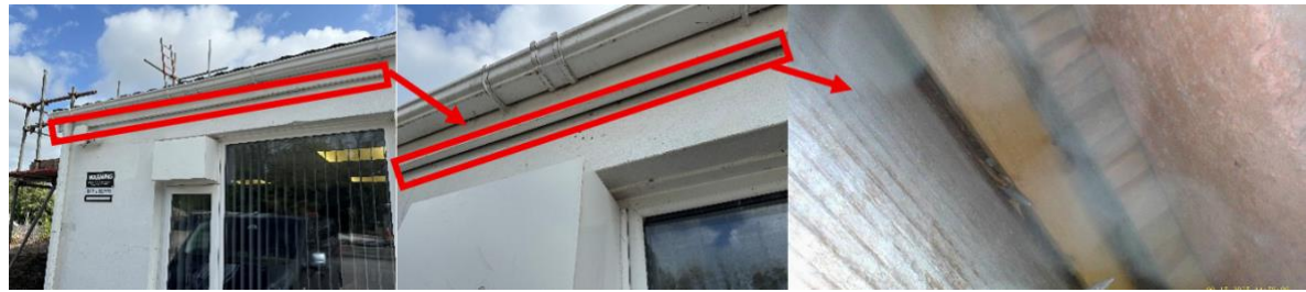
Gaps under fascia boards
