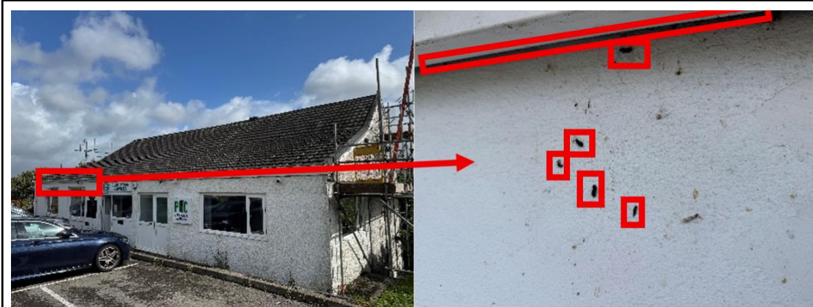
Example of bird droppings found on the front of the building
