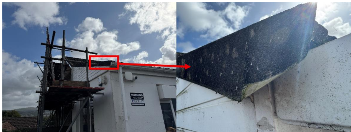
Lifted felt flashing
