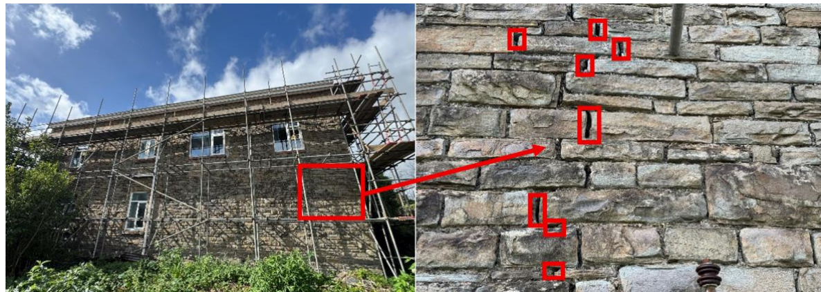
Gaps in stonework
