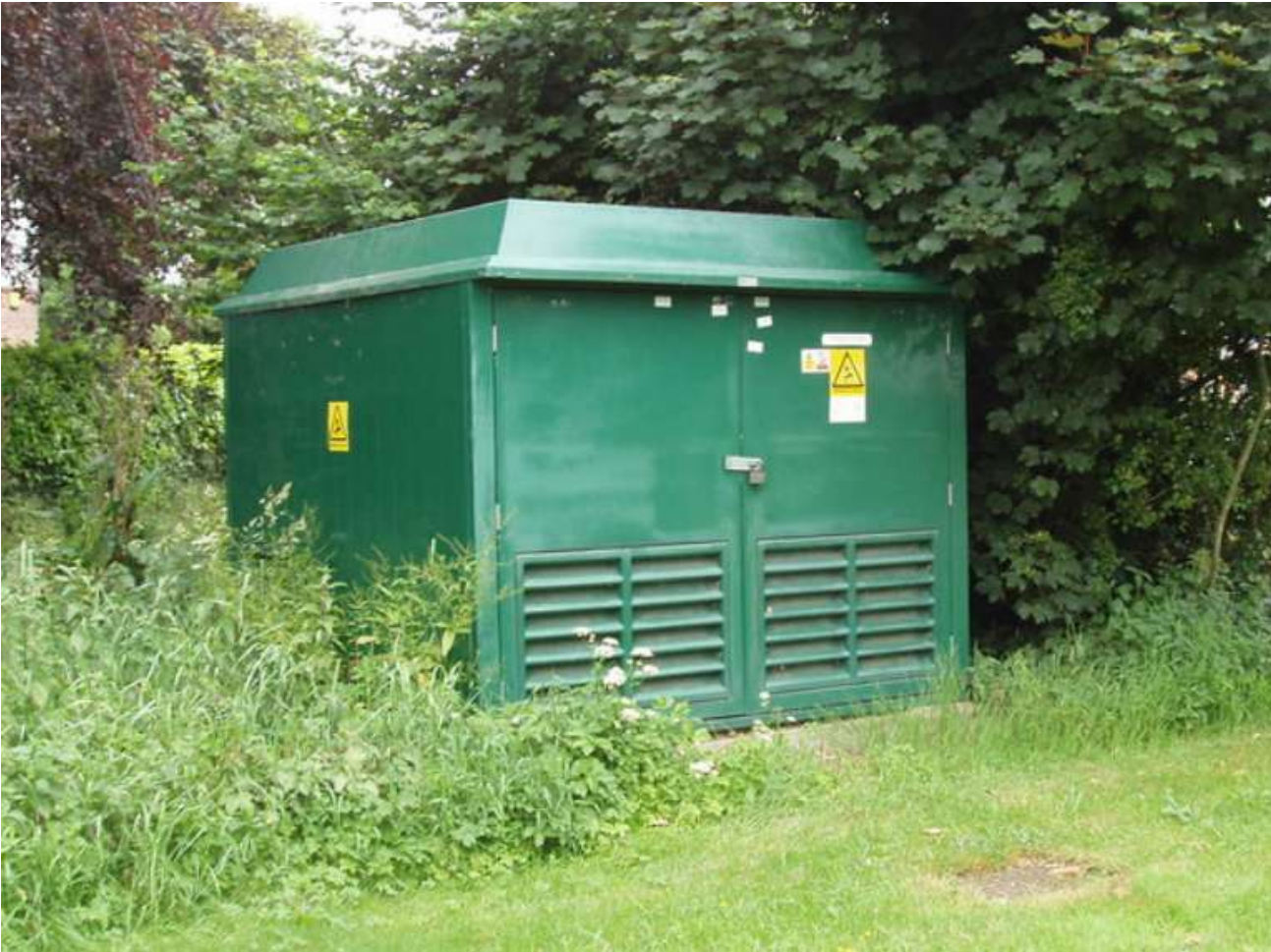
GRP Substation Enclosure
