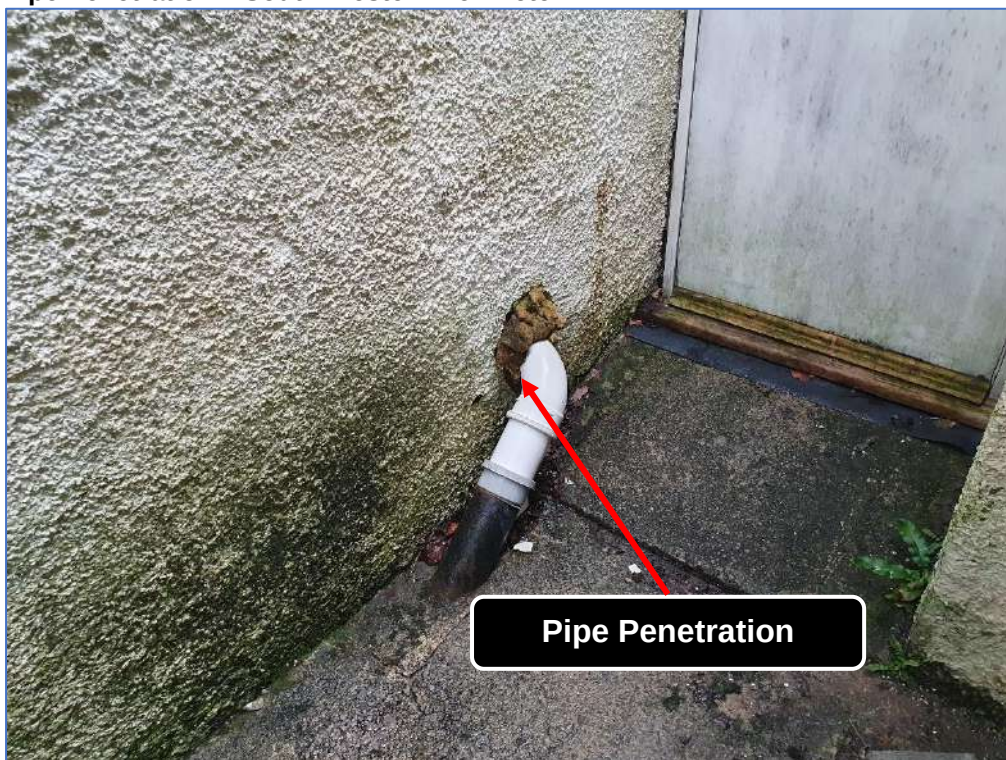
Pipe Penetration – South Western Perimeter
