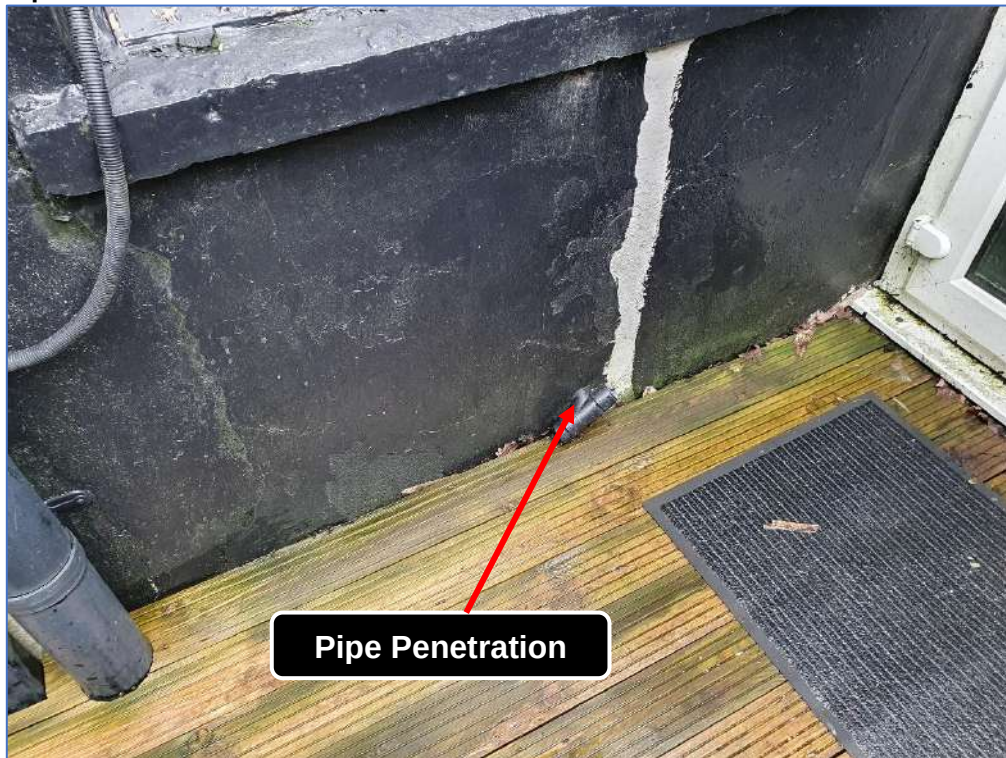
Pipe Penetration – South Western Perimeter
