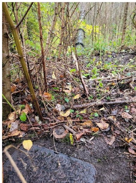
Photo 12: Connection & Overground Section
