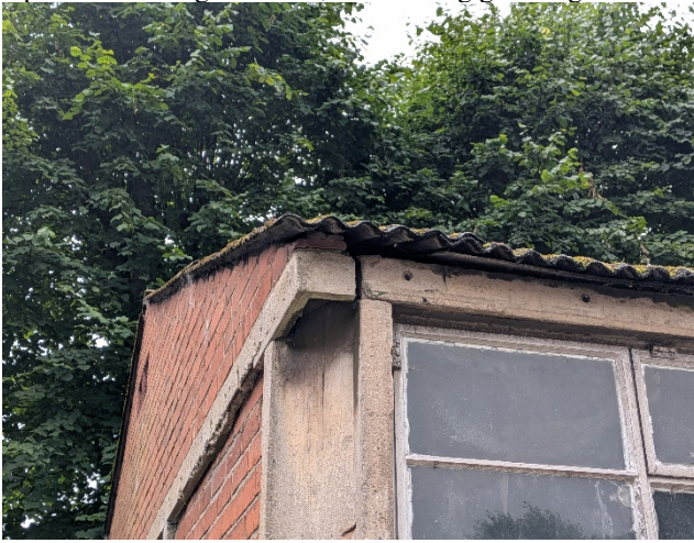
Missing fascia and gaps underneath roof sheeting on B2
