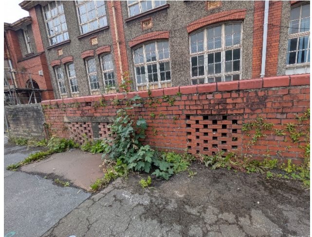
Exterior of subterranean boiler room
