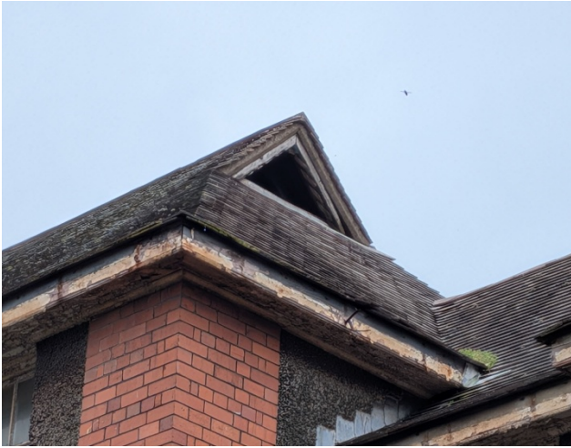
Missing slats and fascia on eastern elevation of B1
