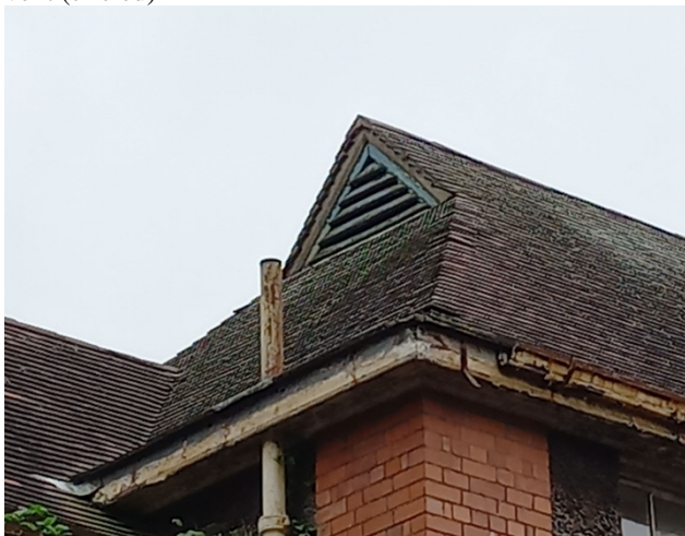
Example of missing fascia and roof vent with open slats on B1
