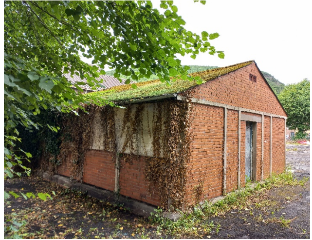
B2 southern elevation with dense ivy growth
