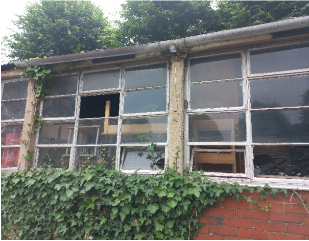
Open and missing windows, and missing guttering on B2
