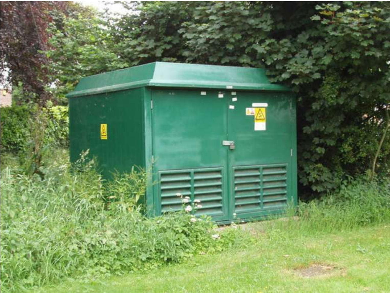
GRP Substation Enclosure
