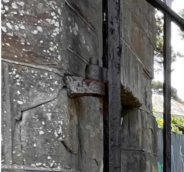
Figure 3, Damage at Hinge Location
