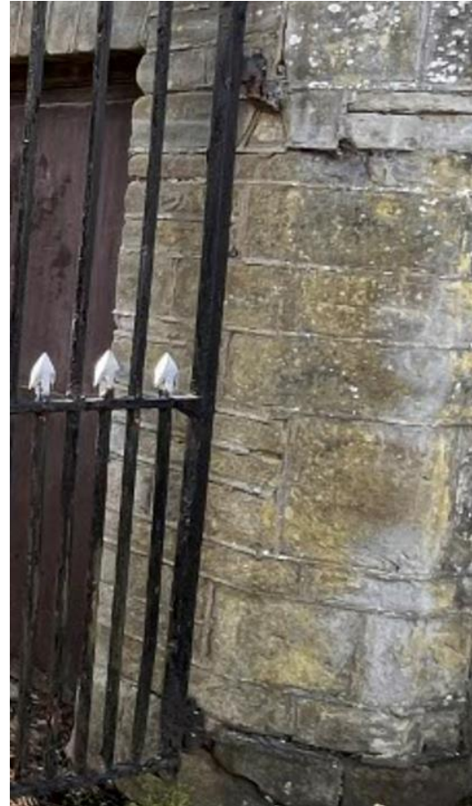
Figure 4, Damage at Hinge Location
