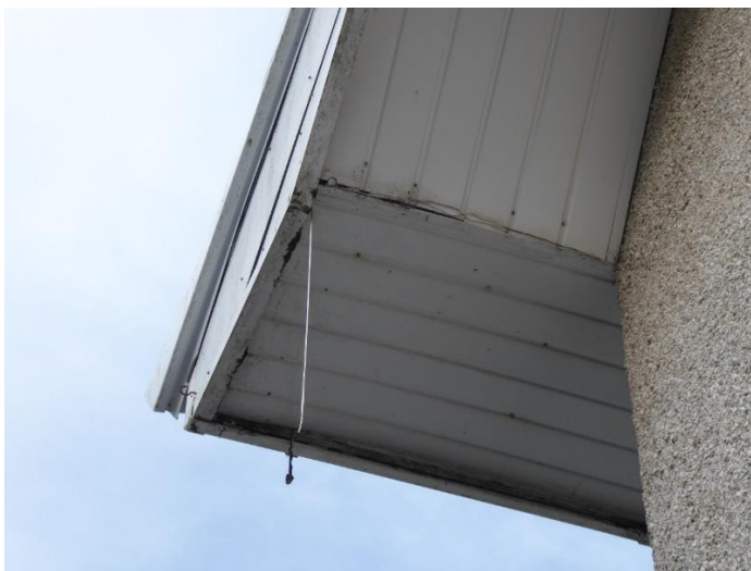
Figure 8 South facing elevation showing gaps at fascia / soffit boards
