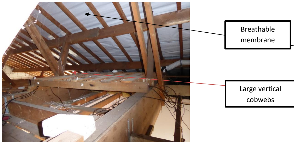
Figure 12 Loft space showing cobwebs
