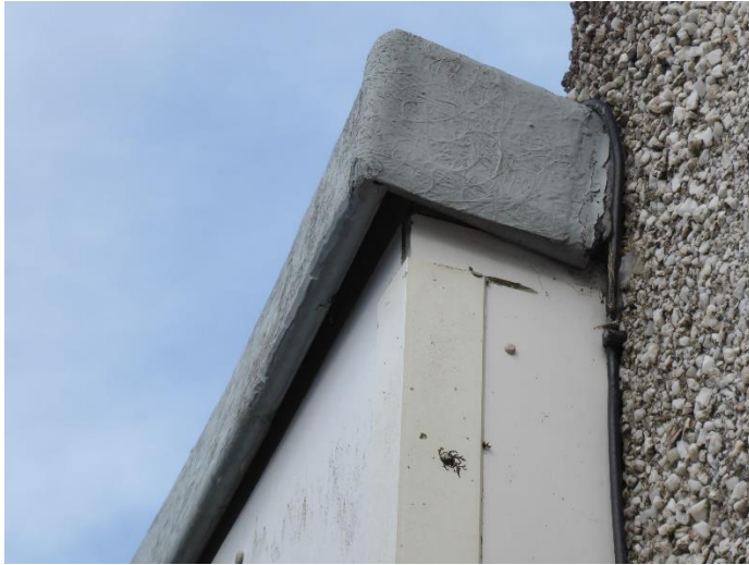
Figure 9 Gaps at flat roof / fascia junction
