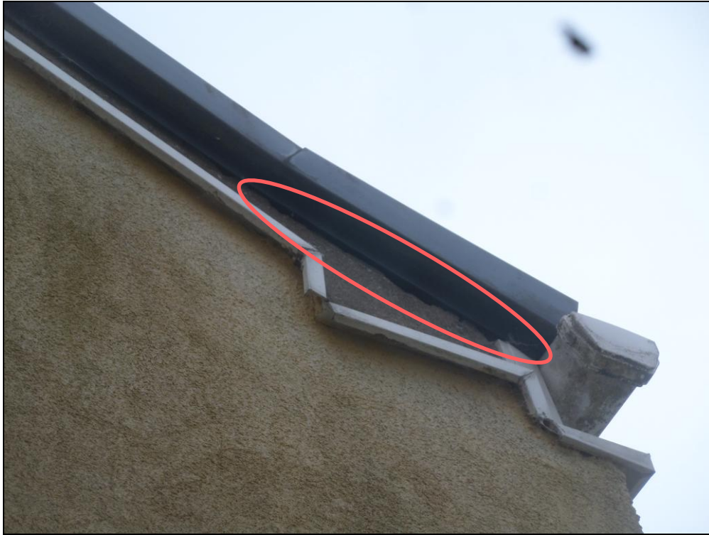
Photo 3: Gap beneath fascia on western gable of southern pitch (view looking south east).
