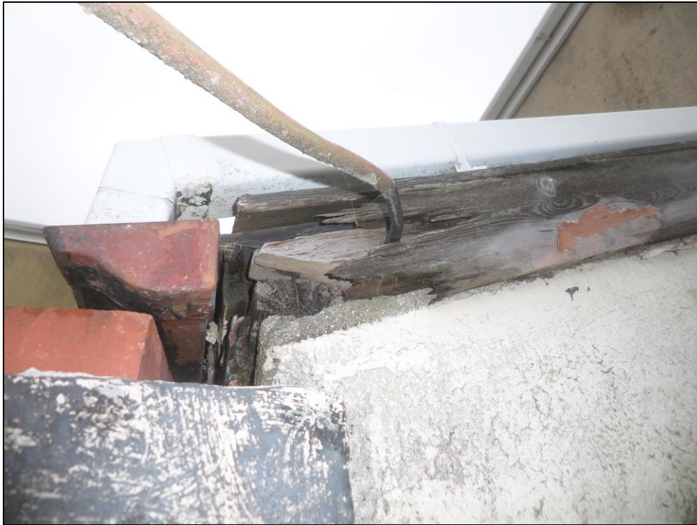
Photo 5: Gap around rotten wooden fascia on southern elevation of southern extension.
