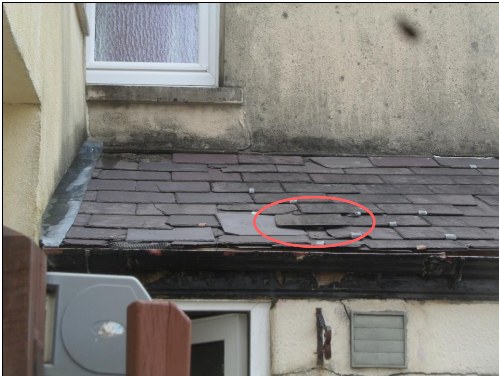
Photo 4: Gap beneath raised slate on southern extension (view looking east).
