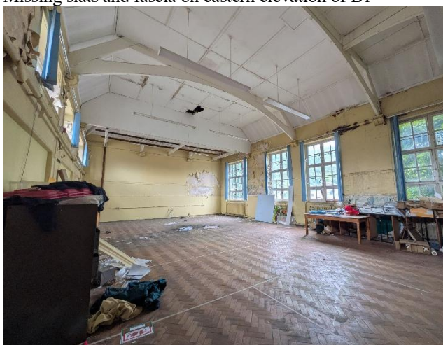
B1 interior, ground floor, large gap in ceiling
