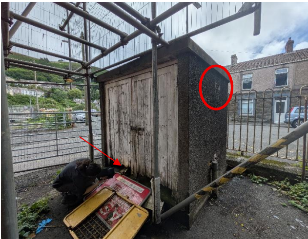
Service outbuilding with gap underneath door (arrow) and vent (circled)
