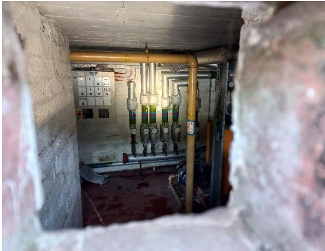
Boiler room interior
