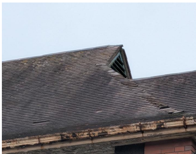
Example of missing and raised roof and ridge tiles on B1
