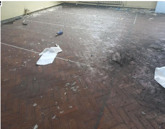
Floor beneath gap with bird feathers and droppings
