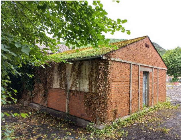
B2 southern elevation with dense ivy growth
