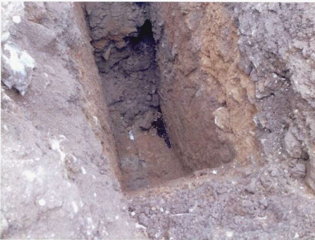
Photo 2 – Ingress of free phase product into LEE pit 2.
