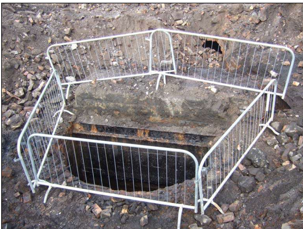
Plate 1 – Tar Tank beneath Unit D.
