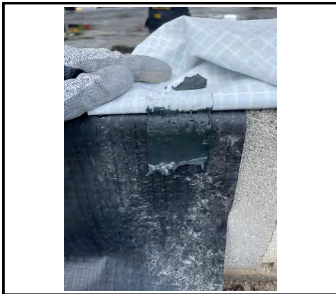
A photograph showing evidence that double sided butyl tape has been used.
