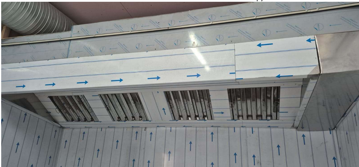
Photo 1: The Commercial Kitchen Extraction Canopy
