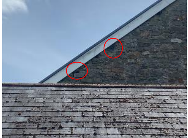
Photo 25: Raised Bargeboard on Northern Rear of Single-Storey Extension, and Gaps within the Stone Masonry (Circled) – B1
