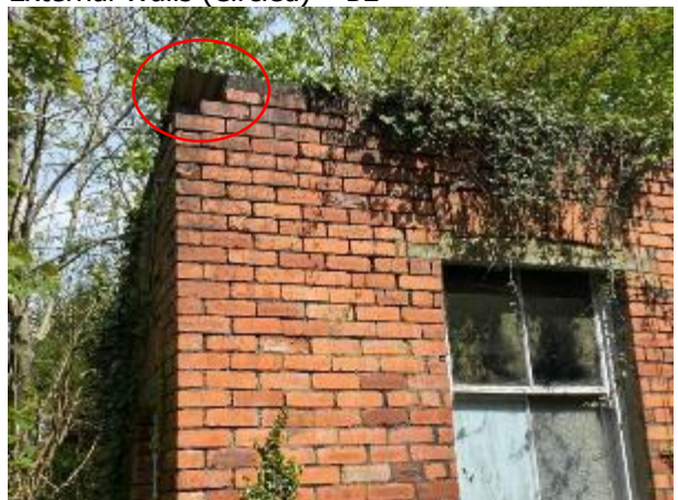
Photo 28 Large Gap Between Corrugated Metal and External Walls (Circled) – B2
