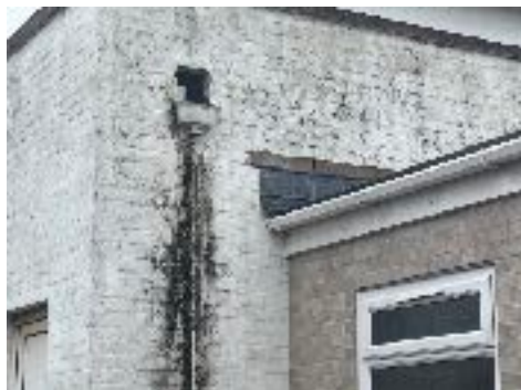
Photo 6. Feature A - gap under lead flashing on northern elevation.
