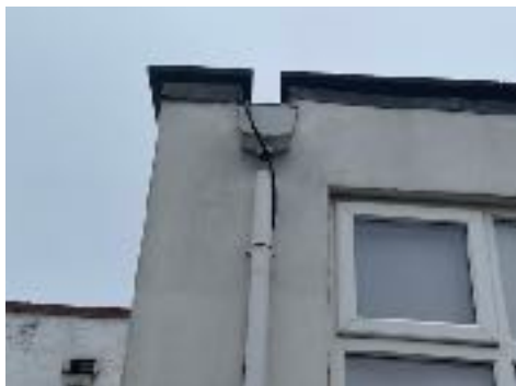
Photo 7. Feature E - gap under fascia of flat roof along corner of building. Fascia bends away from vertical wall slightly.
