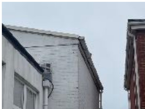
Photo 8. Feature F - gap in corner of plastic soffit of pitched roof.
