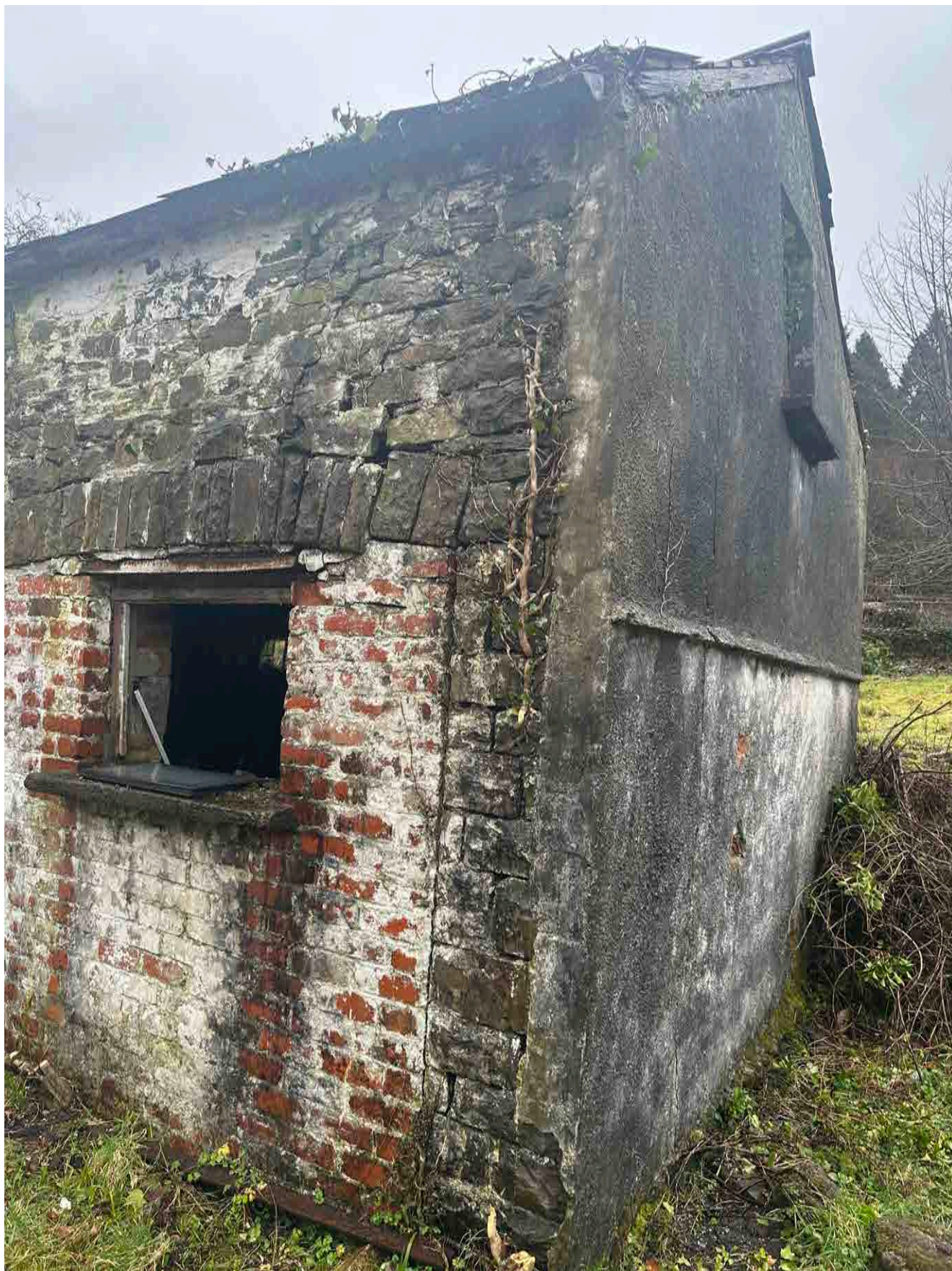
West corner showing leaning brick panel and cracks in the stone masonry above.
