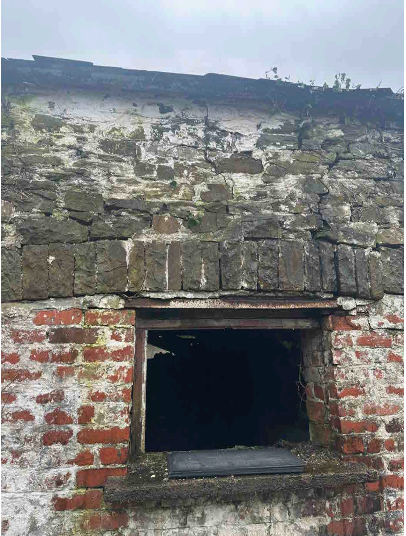
Cracked masonry above opening in the north western face. Repointing is required here once rebuilding of the brick panel is completed.
