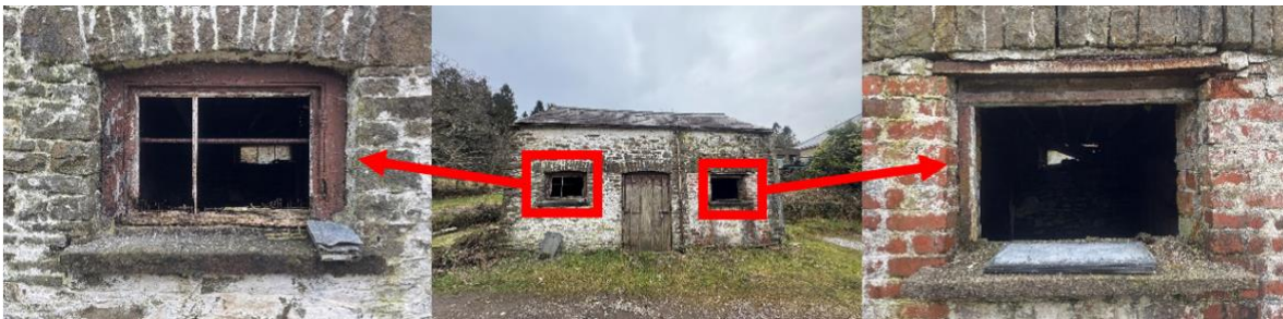
Windows with missing glass on front aspect
