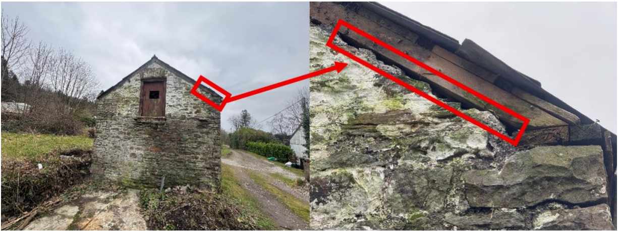
Pipistrelle access point A
