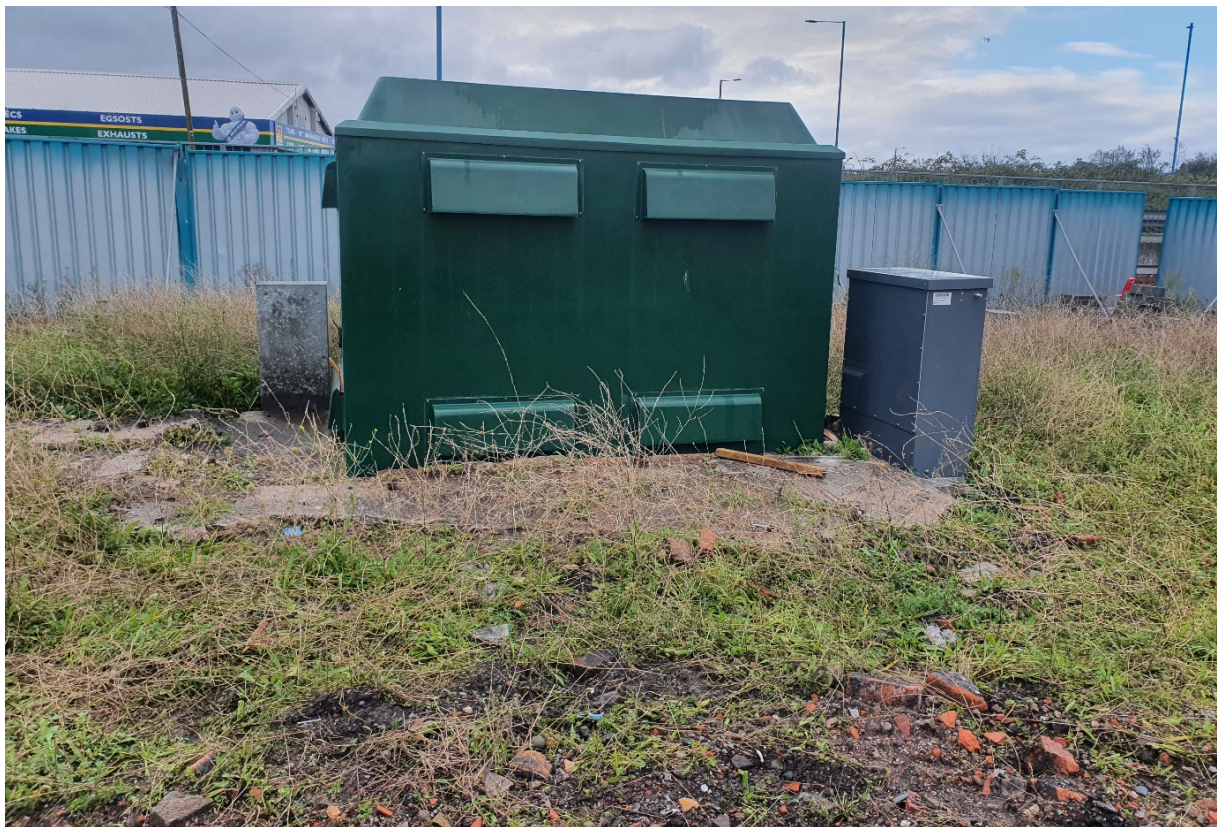
Photograph 4 - Substation in eastern site area.
