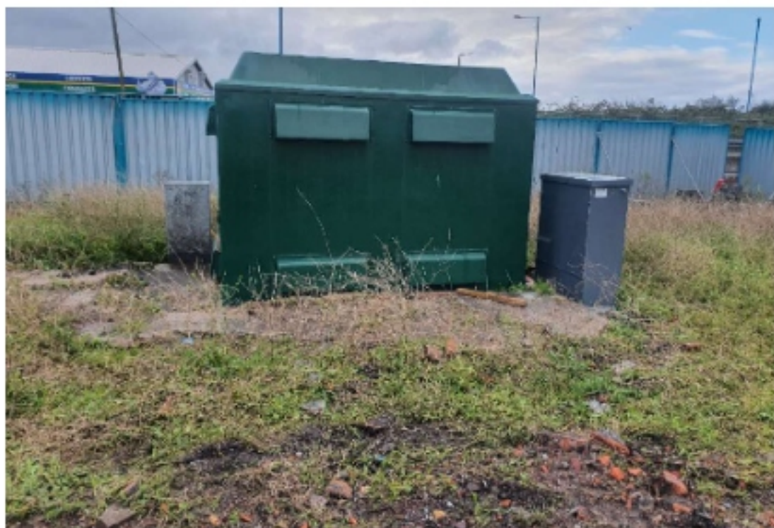
Photograph 4 - Substation in eastern site area.
