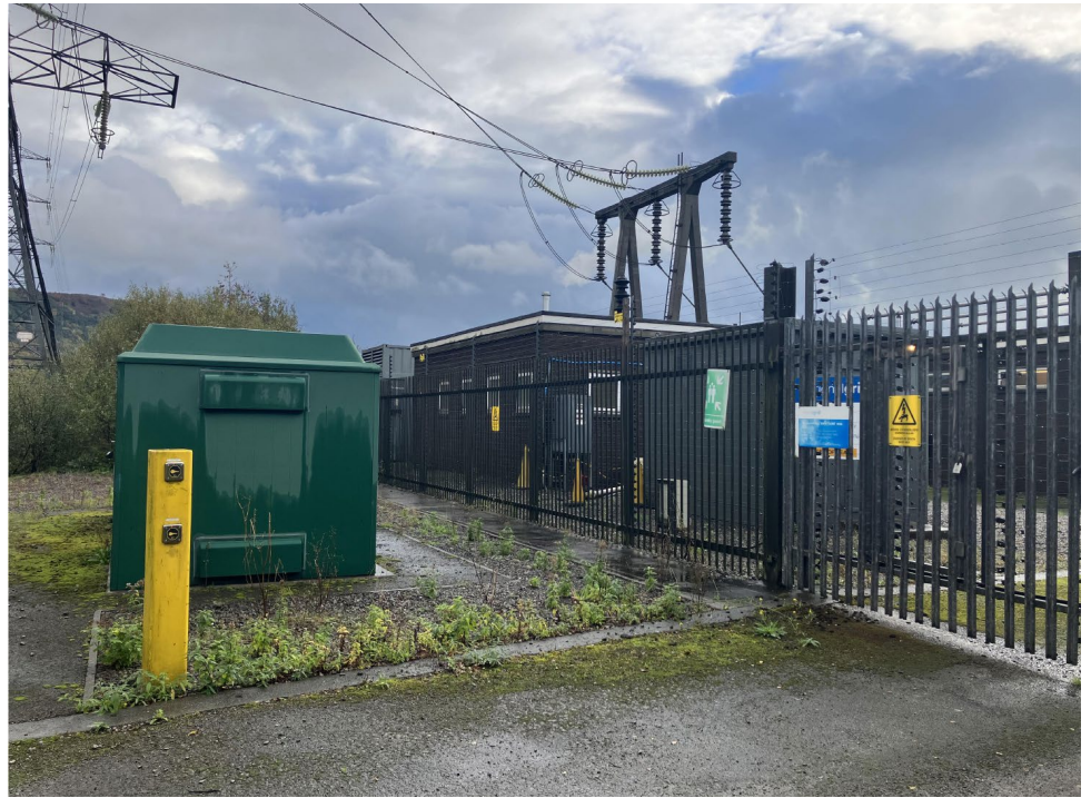
Example image showing steel perimeter fence with electrified wire overhead.
