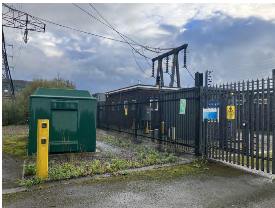
EXAMPLE IMAGE SHOWING PALADIN STEEL PERIMETER FENCE WITH ELECTRIFIED WIRE OVERHEAD. ADDITIONALLY EXAMPLE OF GRP DNO ALSO SHOWN
