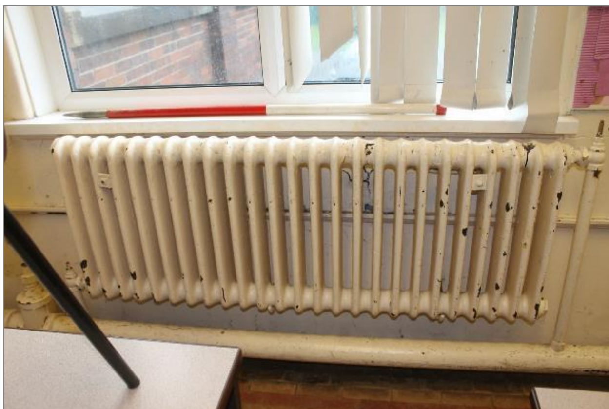
Photo 29: Example of a cast iron radiator in a standard classroom. 1 x 1m scale.
