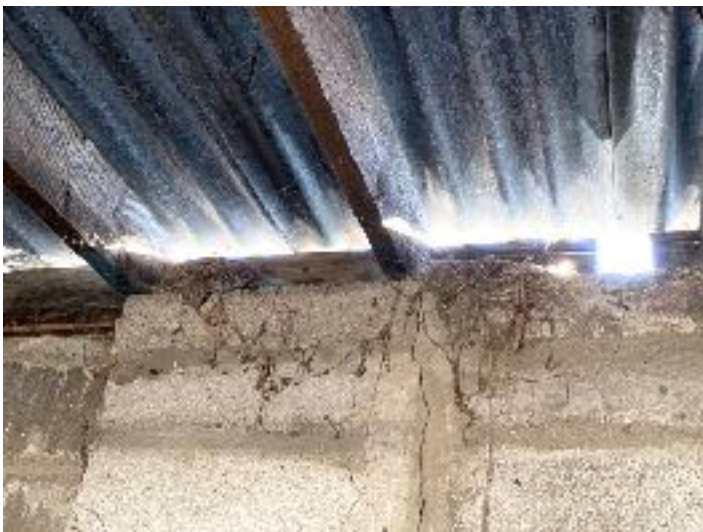
Old Blackbird nests within the block work building on top of the wall plate between the ceiling beams
