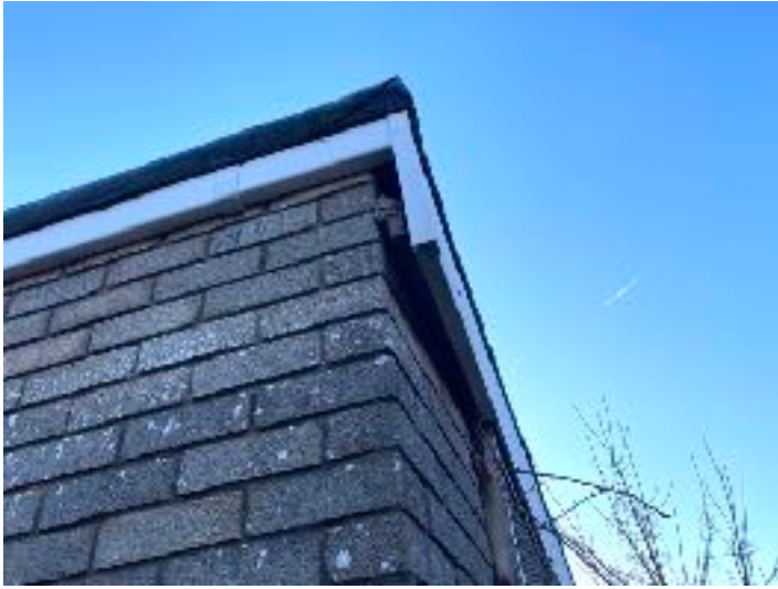
Large gap underneath the barge board at the north west corner of the building
