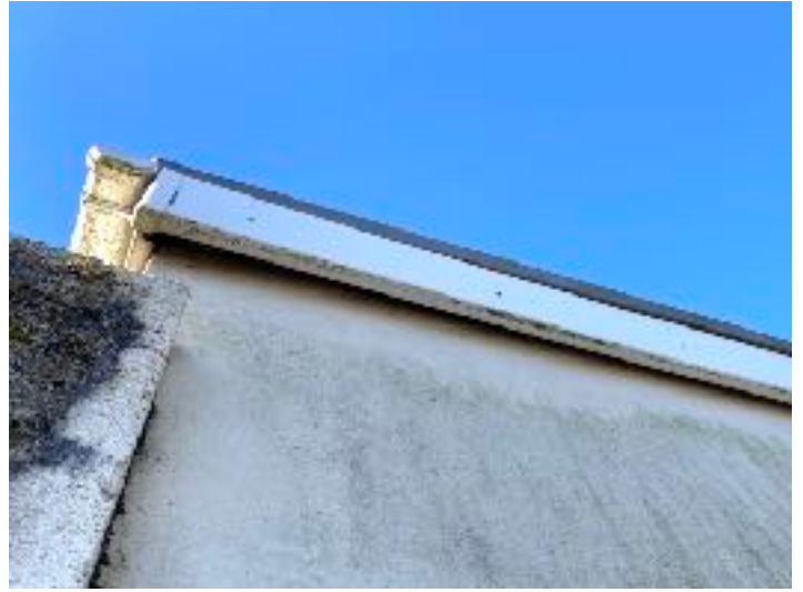
Example of lifted barge board around the former changing room building
