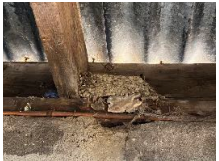
Old Swallow nest within the block work building on top of the wall plate between the ceiling beams
