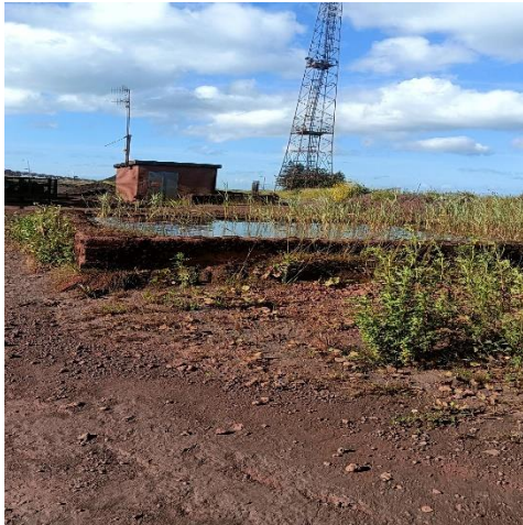
Fig 25 : Vat near conv. 823 & Lighting tower
