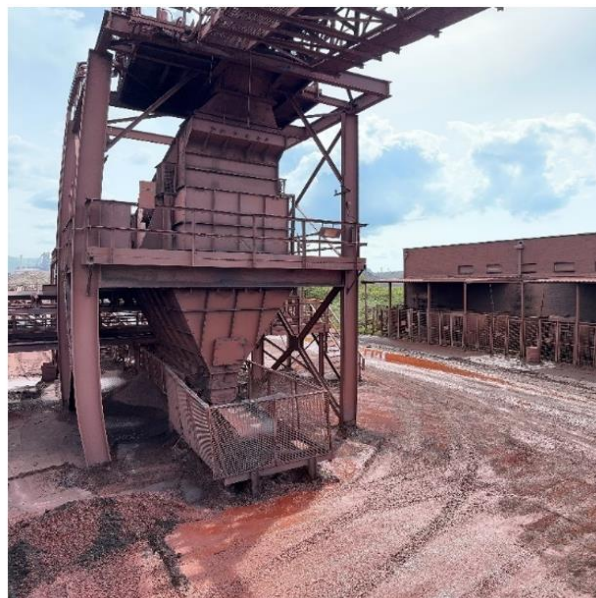
Fig.23 Conveyor 1/831 Loading area
