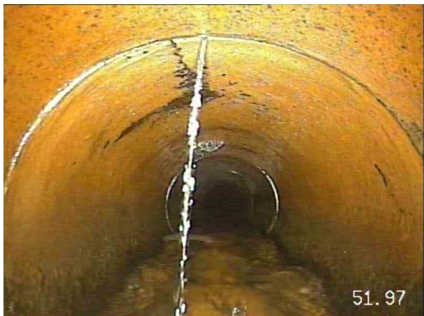
13, 00:13:59, 51.97 m Fracture, longitudinal at joint at 11 o'clock
