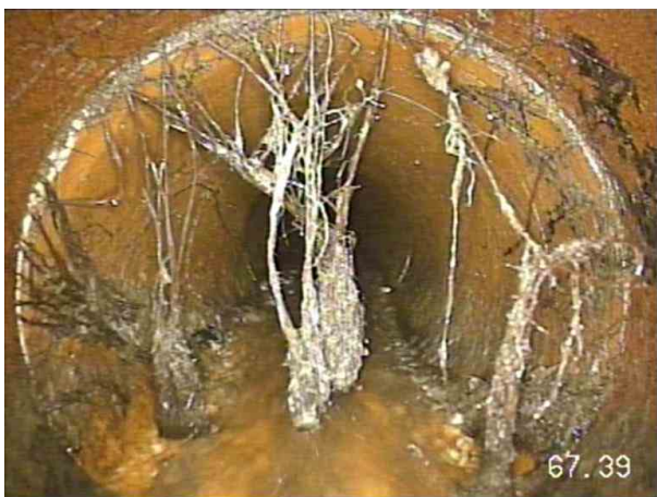
9, 00:11:58, 67.39 m Roots, mass, 10% cross-sectional area loss
