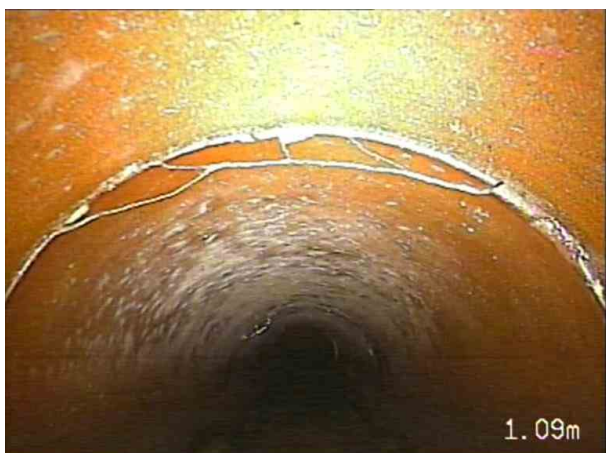
1, 00:00:21, 1.09 m Fractures, multiple at joint from 10 o'clock to 1 o'clock
