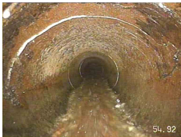
6, 00:09:33, 54.92 m Broken pipe at joint from 8 o'clock to 2 o'clock
