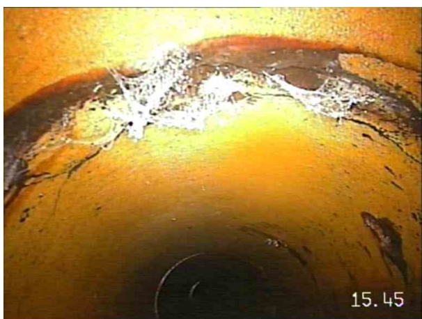
9, 00:05:37, 15.45 m Fracture, circumferential at joint from 10 o'clock to 2 o'clock
