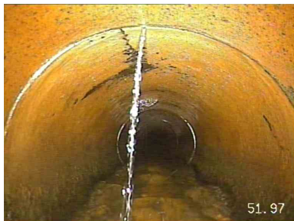
12, 00:13:56, 51.97 m Infiltration, running at 12 o'clock
