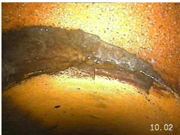
5, 00:03:33, 10.02 m Fracture, longitudinal at joint at 10 o'clock
