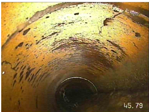
11, 00:12:27, 45.79 m Fracture, longitudinal at joint at 3 o'clock
