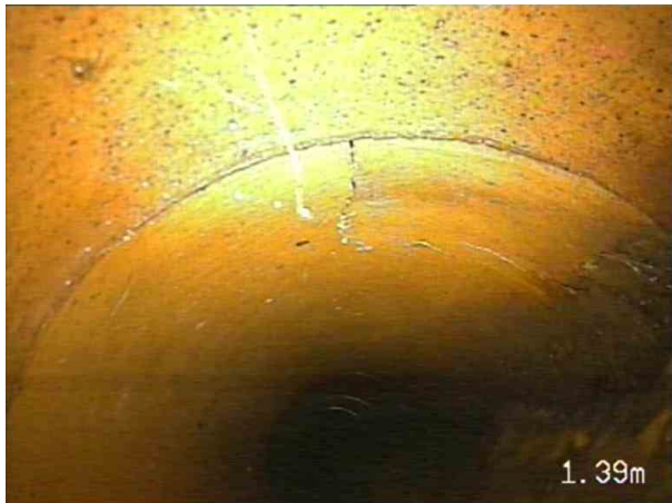
1, 00:00:46, 1.39 m Fracture, longitudinal at joint at 4 o'clock
