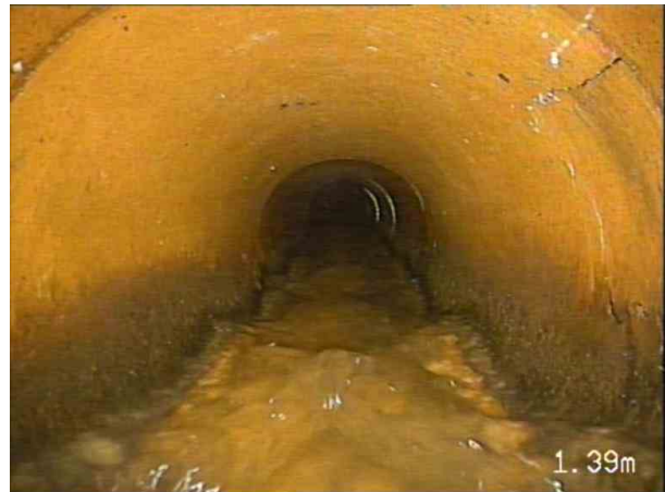
2, 00:00:52, 1.39 m Fracture, longitudinal at joint at 2 o'clock
