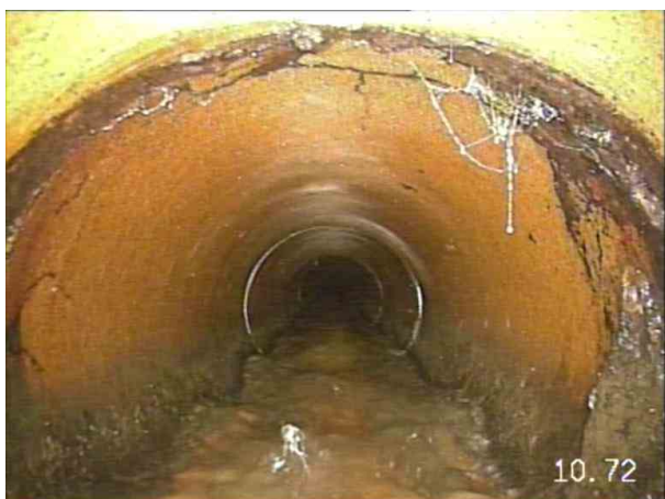
7, 00:04:14, 10.72 m Fracture, circumferential at joint from 9 o'clock to 2 o'clock
