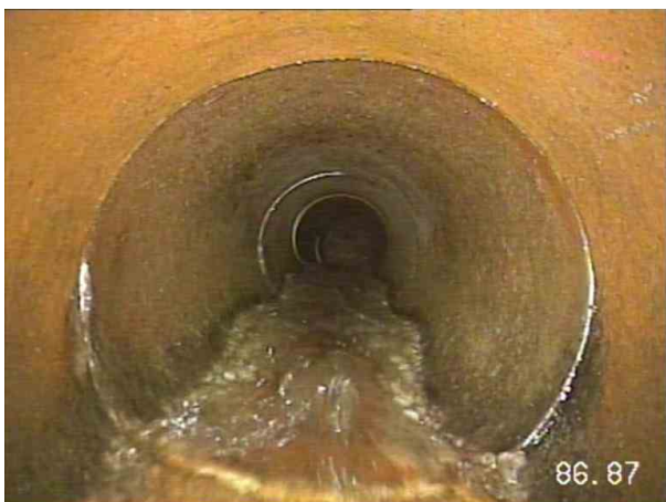
11, 00:14:29, 86.87 m Infiltration, running at joint at 9 o'clock
