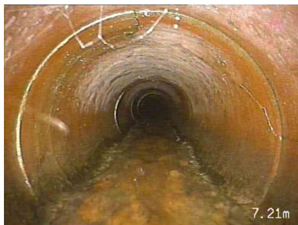
2, 00:01:25, 7.21 m Fracture, longitudinal at joint at 12 o'clock
