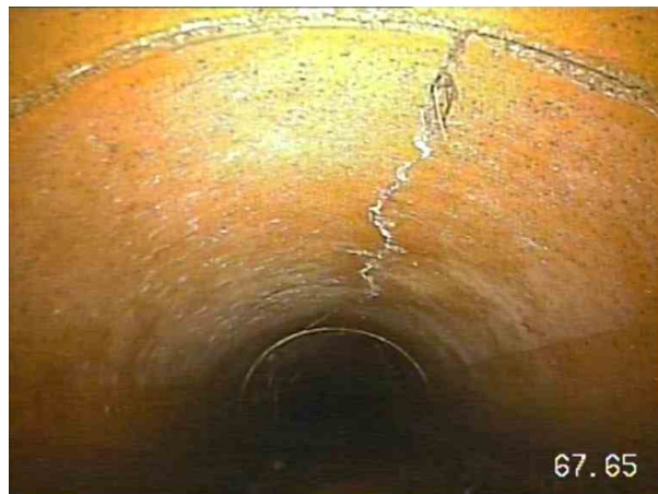
14, 00:16:59, 67.65 m Fracture, longitudinal at joint at 12 o'clock
