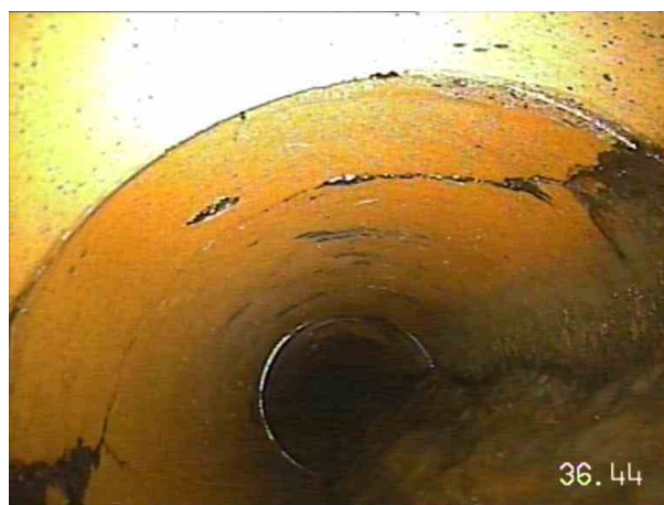
10, 00:10:36, 36.44 m Fracture, longitudinal at joint at 3 o'clock
