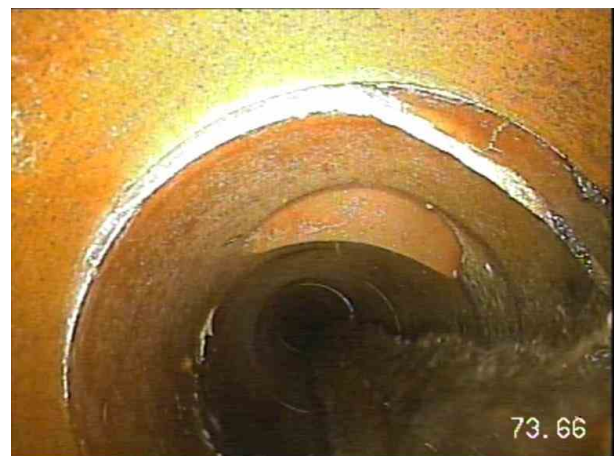
10, 00:12:56, 73.66 m Broken pipe at joint from 2 o'clock to 5 o'clock
