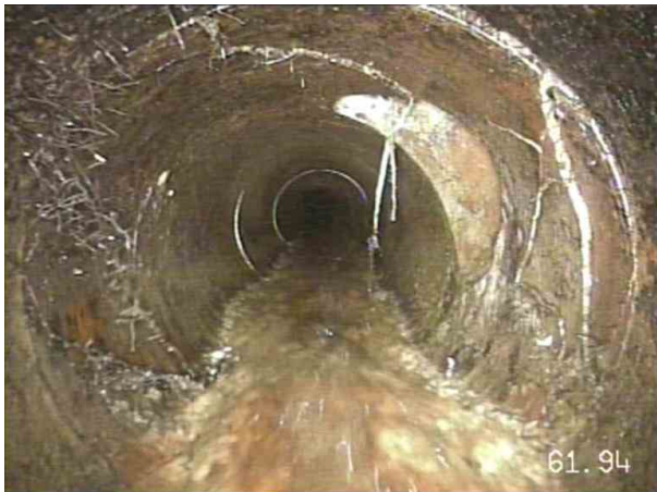
7, 00:10:41, 61.94 m Broken pipe at joint from 2 o'clock to 4 o'clock
