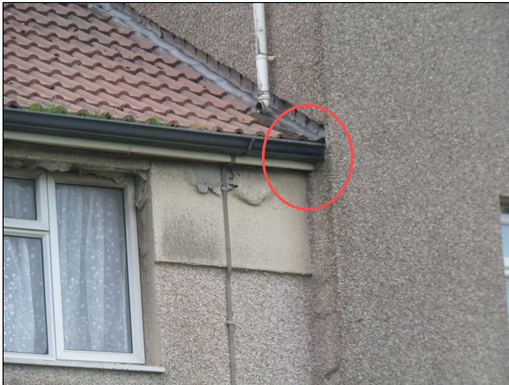
Photo 15: Location of House Sparrow in soffit of Carmarthen House.
