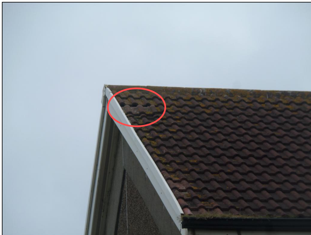
Photo 7: Dislodged roof tile on eastern pitch of southern complex arm (view looking west).
