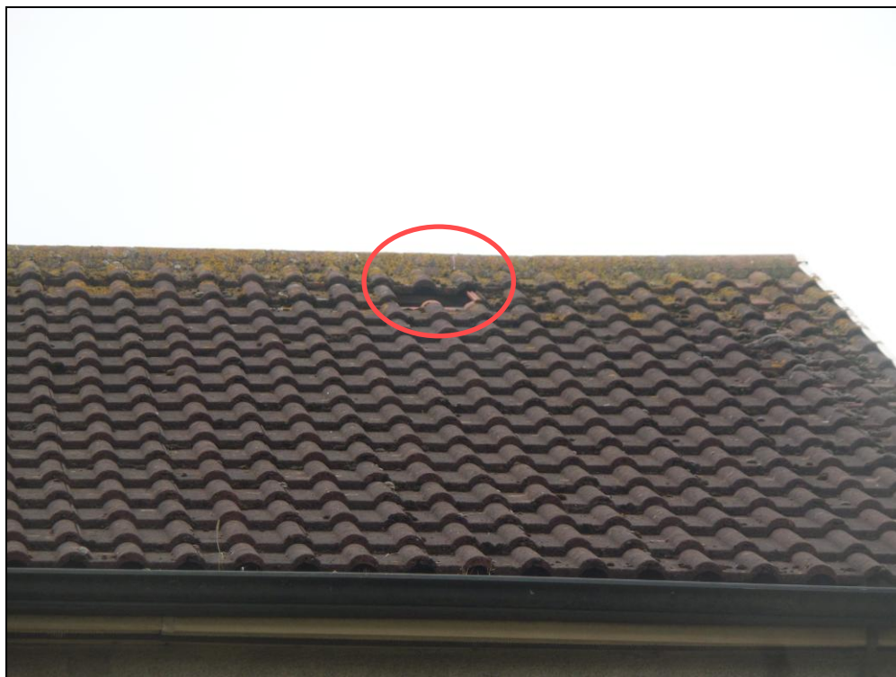
Photo 8: Missing roof tile on northern pitch of western complex arm (view looking south).
