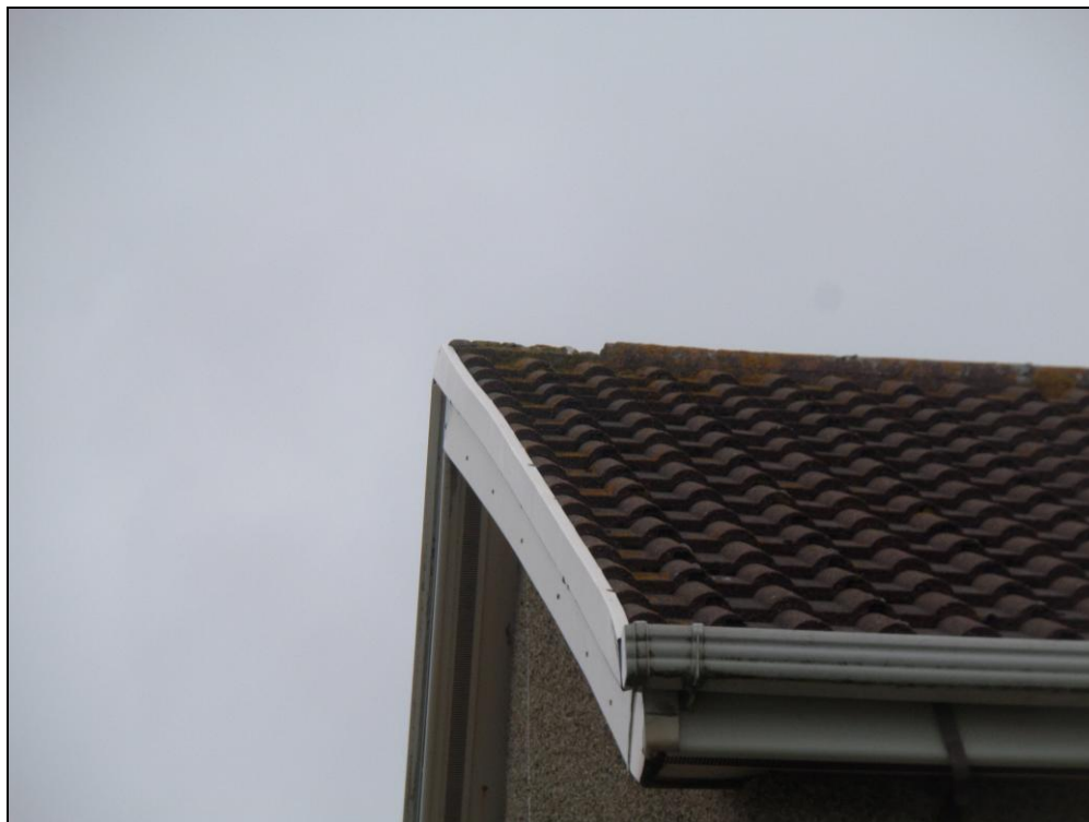
Photo 10: Missing ridge tile located on western gable end of Cardigan House (view looking north).
