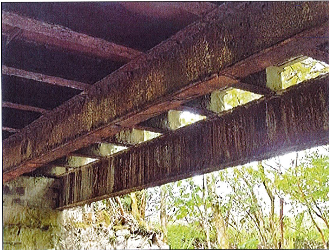
Photo Four Closeup of the central main beam. This beam has a great deal of corrosion particularly to the bottom flange. This will reduce the load carrying capacity. The other steelwork has some surface corrosion which is not significant.
