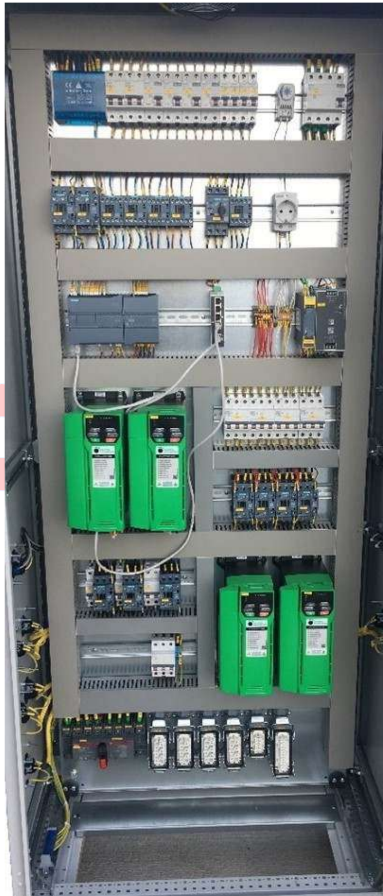
Picture 11. Ferris Wheel Electric Control Panel
