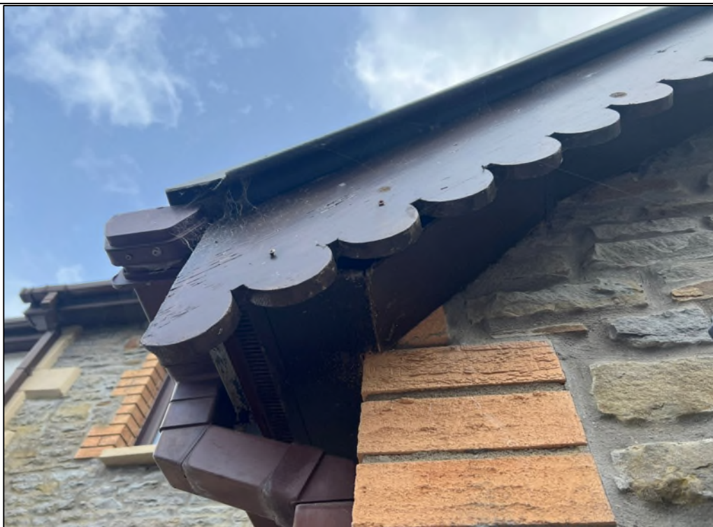
Plate 9 - Gaps between the soffit and fascia where birds have been reported to have nested.
