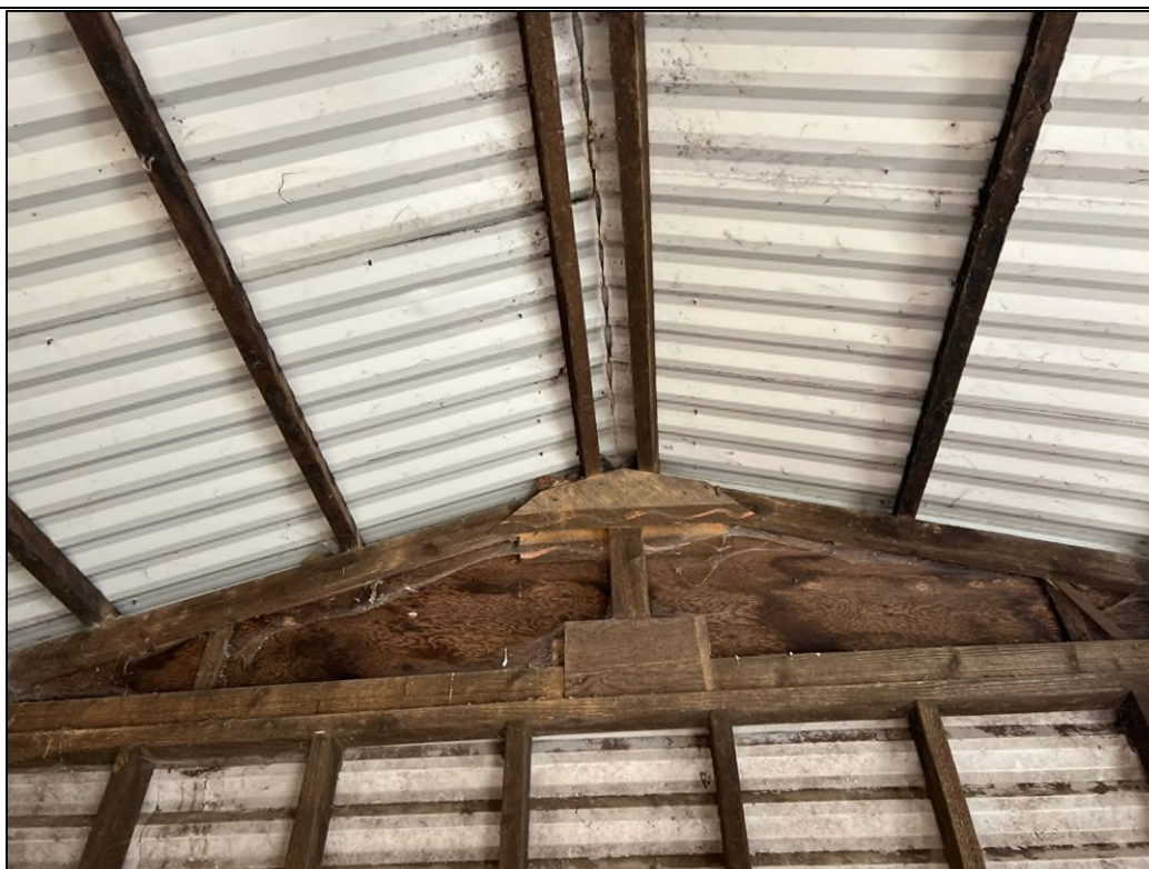
Plate 12 - Inside of the stables due to be demolished with previous evidence of bird nests.
