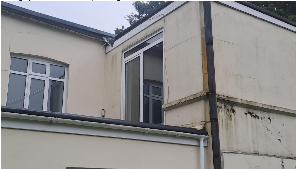
Photograph 6 – Rear elevation, cracking
