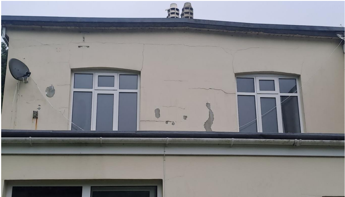
Photograph 5 – Rear elevation, cracking
