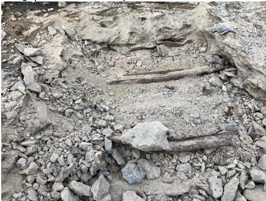
Photograph 24 – Corroded steel within roof structure
