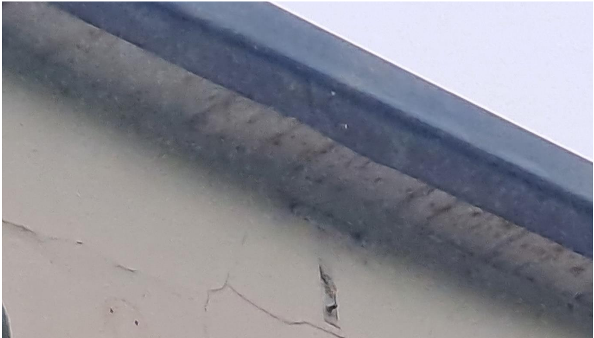
Photograph 11 – Corrosion staining to steel reinforcement within the roof
