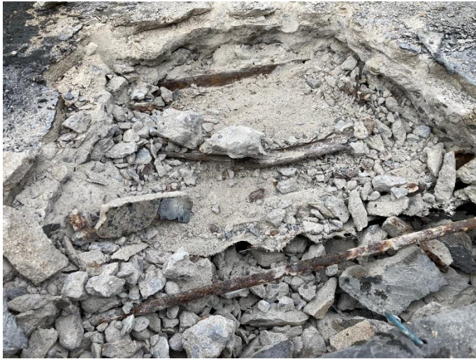
Photograph 25 – Corroded steel within roof structure
