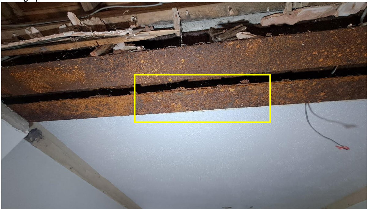
Photograph 14 – Section loss corrosion to steel beams supporting rear of property
